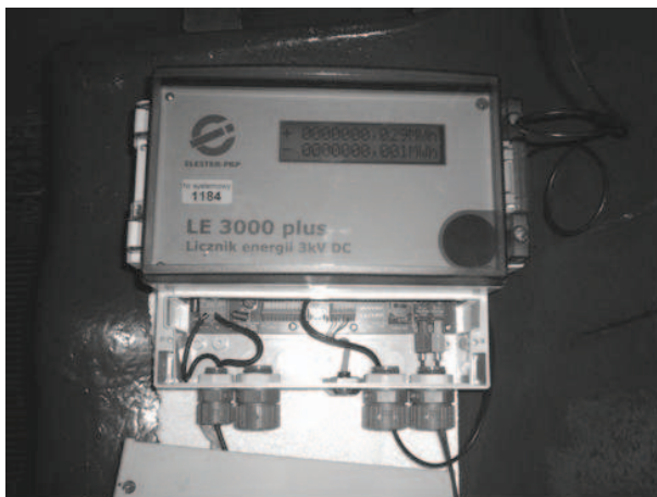
Fig.1. Current electricity meters used in measurements
