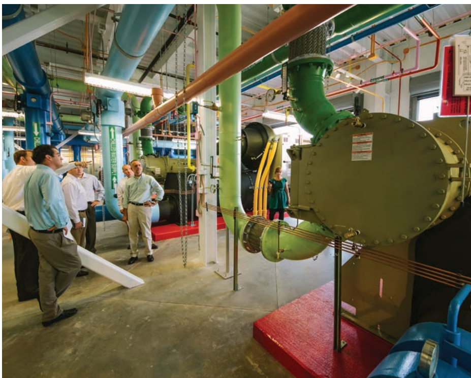
University community members view the Central Energy Plant's color-coded piping and equipment that provide chilled water for air-conditioning throughout campus.
