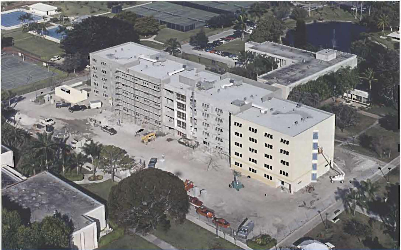
Construction continues on the new E.M. Lynn Residence Hall, which is scheduled to be open for students in September 2002.
