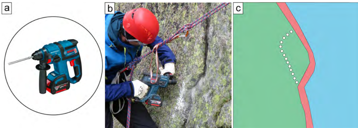
Figure 8.4: (a) Example of a battery powered rotary hammer (GBH18V-26K24 Bosch model). (b) Picture of a surface sample along the Moine transect. (c) Schematic of the sample surface showing the surface of interest (in green), the free surfaces (in red), the unwanted surface (in blue) and the drill holes (white dots), which should be later punched with a chisel and hammer to propagate the fracture and collect the sample.
