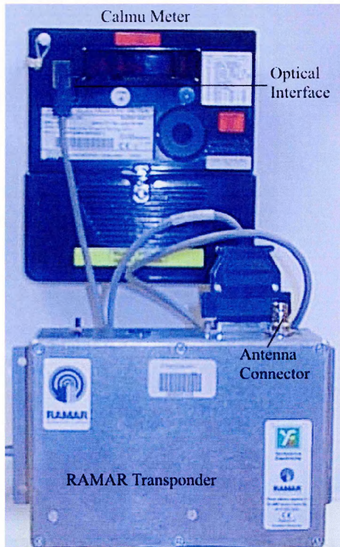
Figure 44 Calmu multi-phase electricity meter and Yorkshire Electricity Group PLC Transponder
