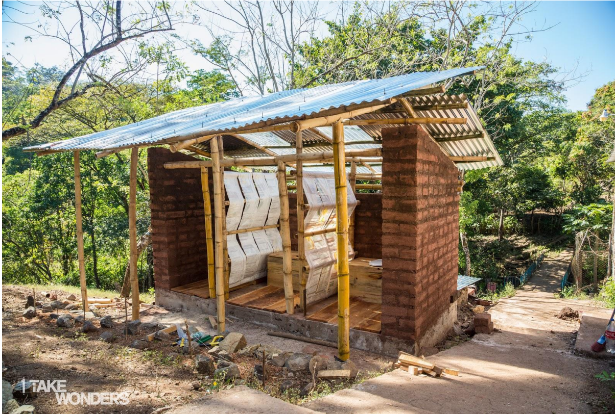
Fig.2 – Progress of the building site at the end of the 12th week of the project (courtesy of Justin Bench).
