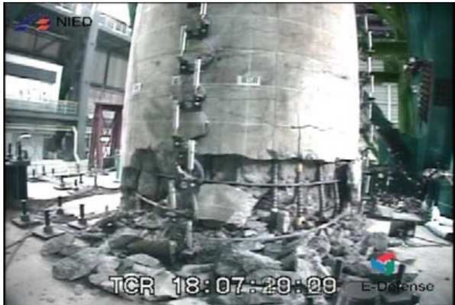
Figure 6-82: Damage to RC pier after 2nd 100% Takatori excitation [1] (2007-1213-014-1M)
