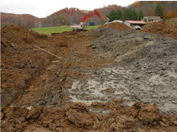
Figure 6. Construction of cross-valley groundwater dam at Mill Branch. Gray, organic-rich gravel and wetland soils were removed and placed on the surface. Brown, clayey silt was placed and compacted in a trench to form the groundwater dam.
