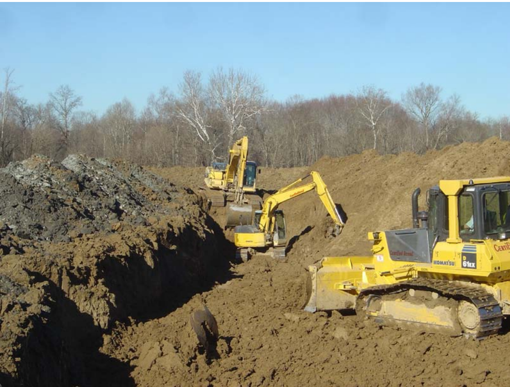
Heavy equipment is used in the restoration process at Dix River in Lincoln County, Kentucky.
