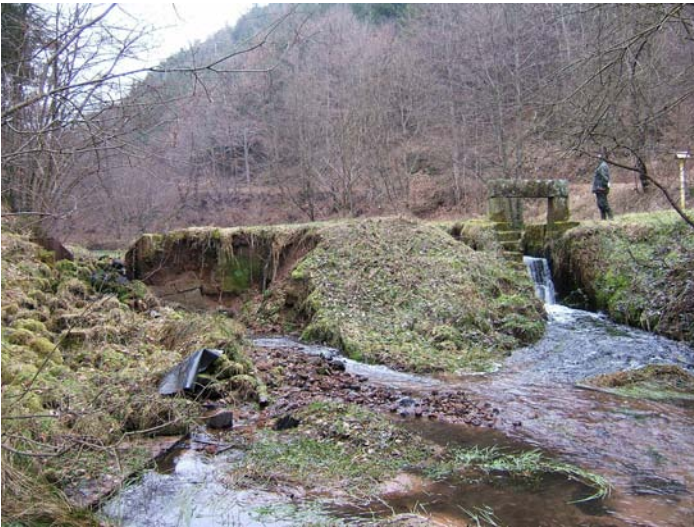
Figure 11. Drift pond dam from the 19th century with historical outlet structure (right side) and damage requiring restoration (left side)
