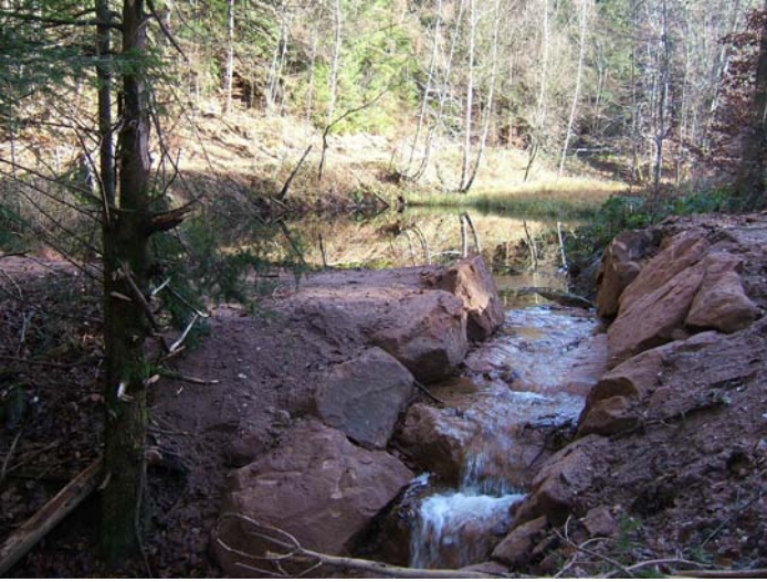
Figure 10. New outlet construction formed as an overfall with cascades into the tailwater
