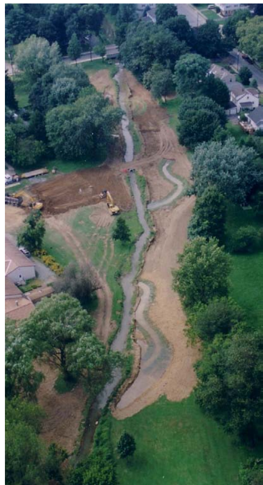
Figure 7. Santo Domingo Creek in New Street Park, Lititz, PA - During Construction. Aerial view shows the new, meandering channel under construction as water continues to flow through the existing straightened channel.
