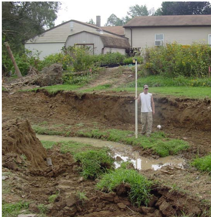
Figure 8. Santo Domingo Creek in New Street Park, Lititz, PA - During Construction. The man is standing on restored floodplain, now attached to the restored channel. The old floodplain elevation, created by the deposition of legacy sediments, can be seen behind him.
