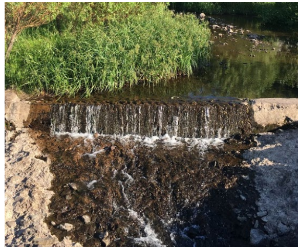
The Lakeshore weir, a 2.5ft high concrete broad crested weir, looking upstream.
