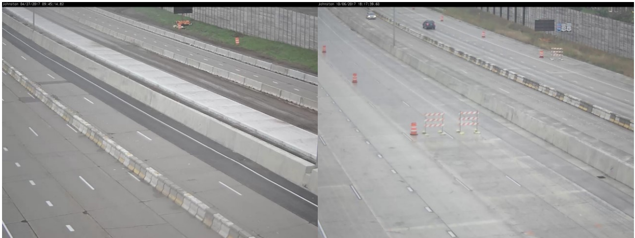
Figure 5.3 Johnson Pkwy Station. Reduced Lanes Layouts. 2-Lane Narrow Through only, 3-Lane Narrow.
