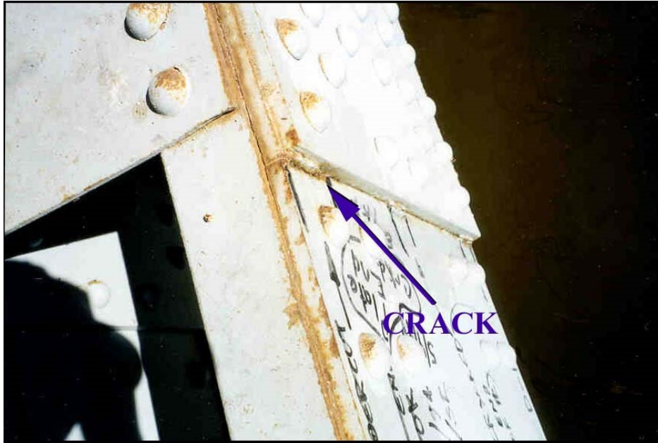
Figure 2.2 Fractured tie girder plate, Hastings Bridge (Niemann, 1999)
