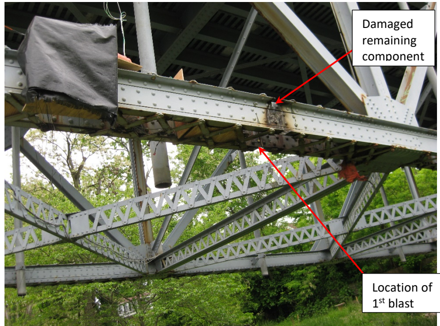
Figure 2.4 Partially severed FCM, Milton Madison Bridge approach span
