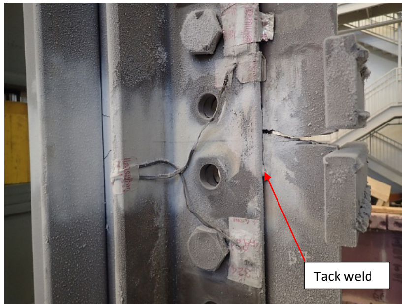
Figure 3.14 Fractured tack weld and center plate
