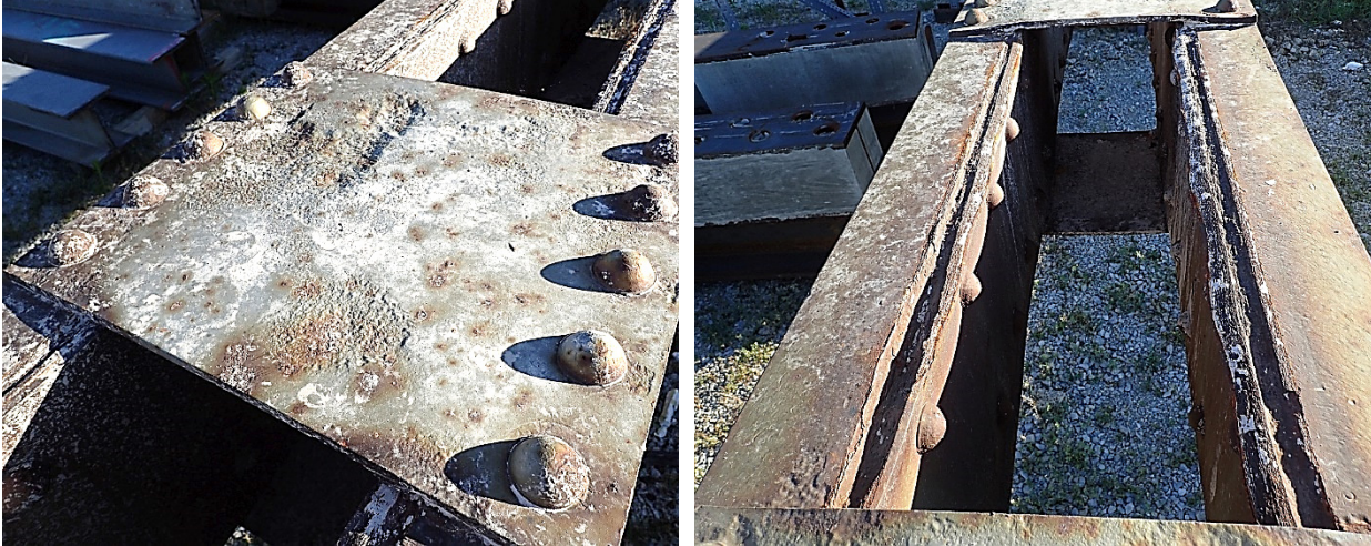
Figure 3.16 View of corrosion damage resulting in section loss and pack rust
