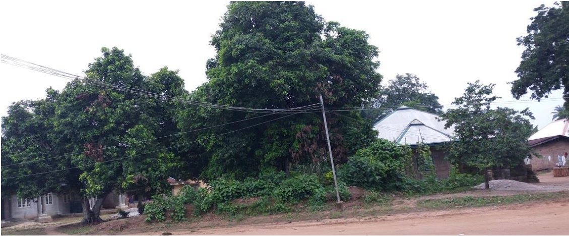
Figure 5.20: Low Voltage Lines supplying Community Homes at Umuagwu Community
