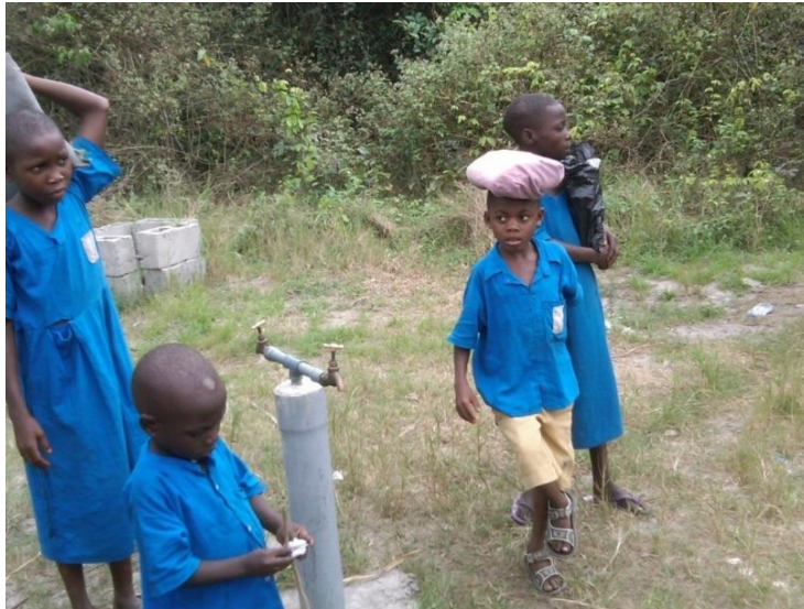
Figure 5.5: Dry Taps at the Elementary School
