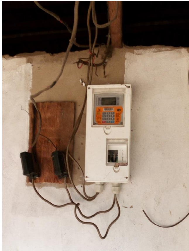
Figure 5.24: Pre-paid Meter Unit at a Consumer's Premises
