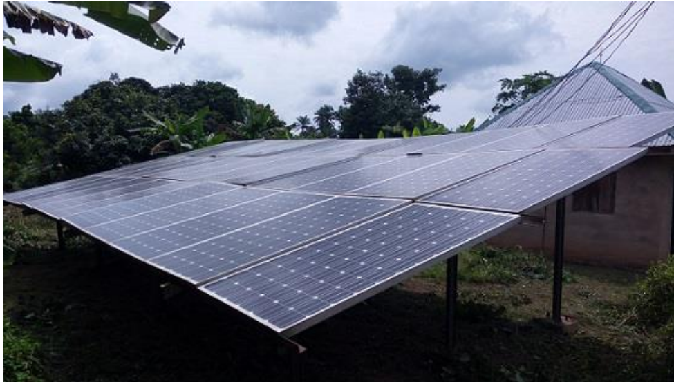
Figure 5.26: Solar Array at Umuode Community
