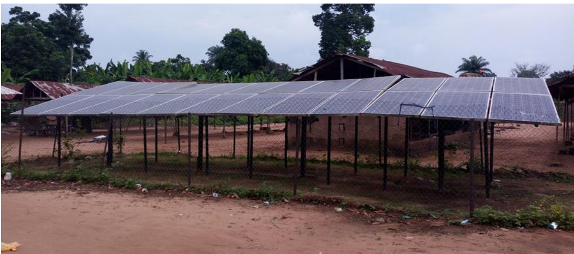
Figure 5.21: The Solar Array at Umuagwu Community
