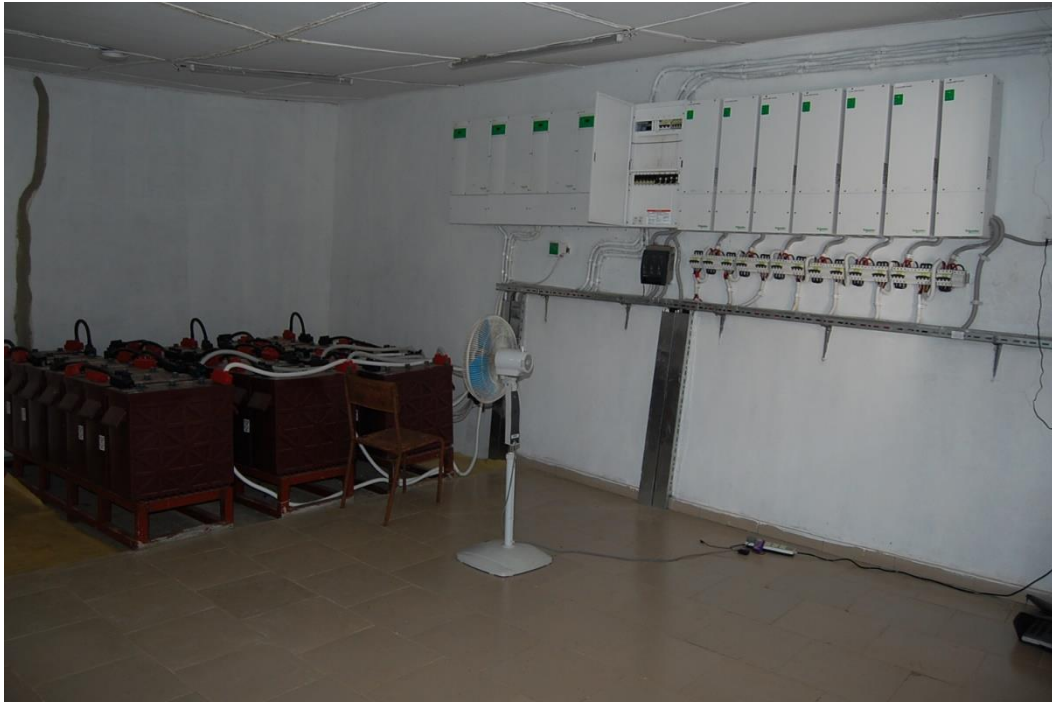
Figure 5.19: The Control Room and Balance of System Equipment
