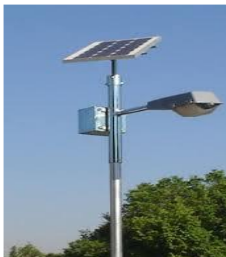
Figure 2.4: A Solar Street Light Installation
