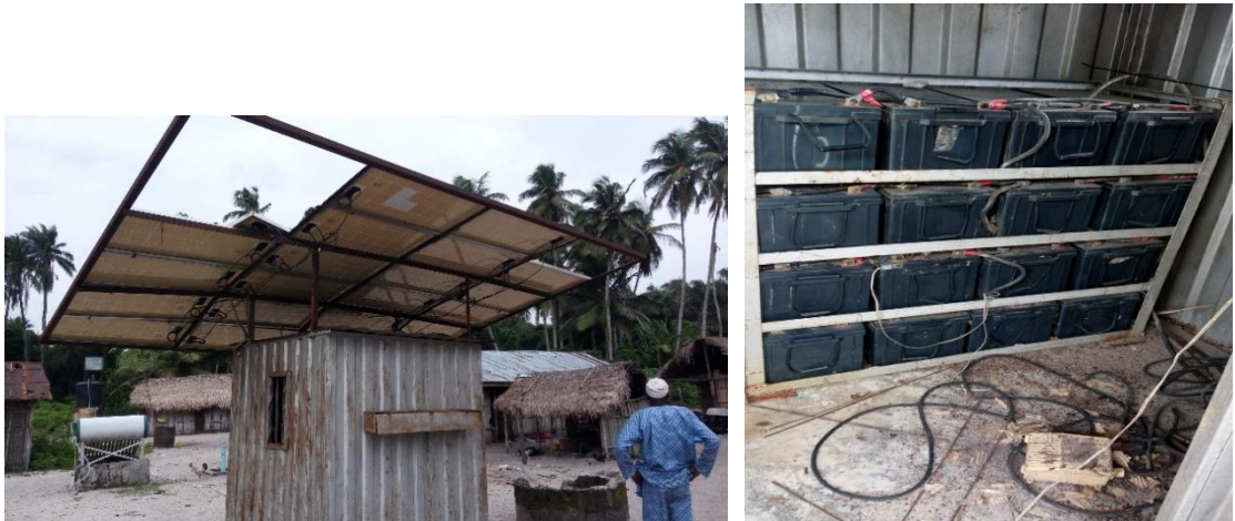
Figure 5.13: Dilapidated Solar panels and Bank of Batteries
