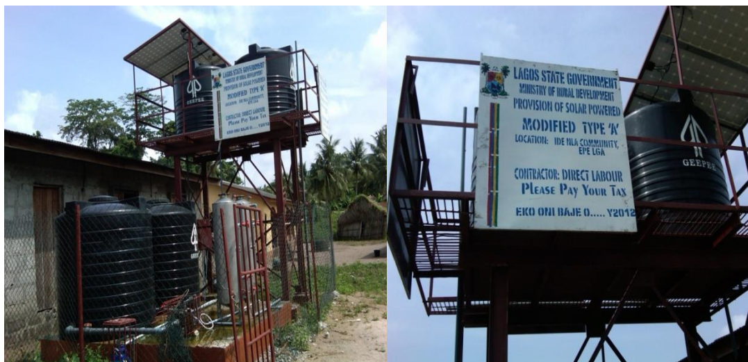
Figure 5.4: Community Solar Water Installation at Ide I Village
