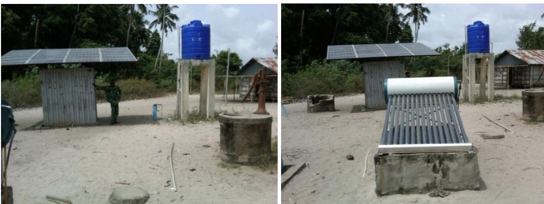
Figure 5.11: Solar borehole system at Ide II Settlement
