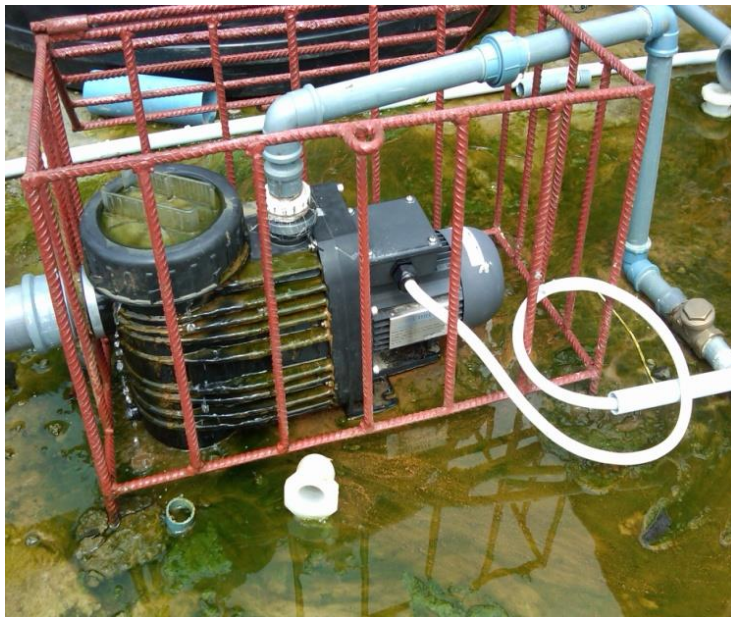
Figure 5.8: Leaking Surface Pump at Ide I Village
