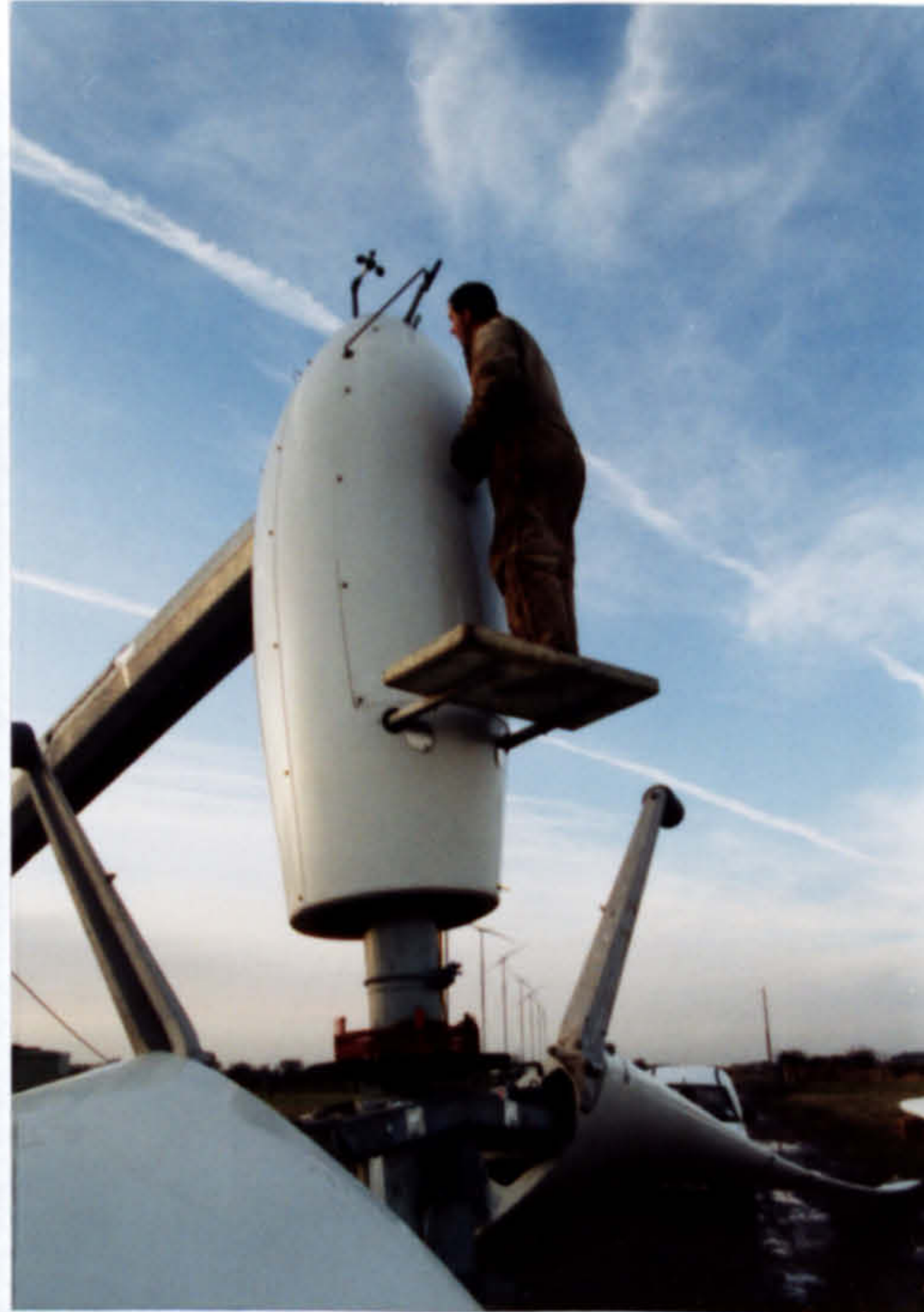
Figure 4.4: Access to the powertrain and other components housed in the nacelle is via a hatch in the GFRP pod.
