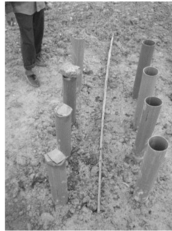
Figure 4.28: The inlets and outlets of PVC pipes buried at 0.5m, 1.0m, 1.5m and 2.0m.
