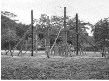
Figure 4.29: Construction of an experiment shed containing the equipment and earth pipe in/outlets commenced.
