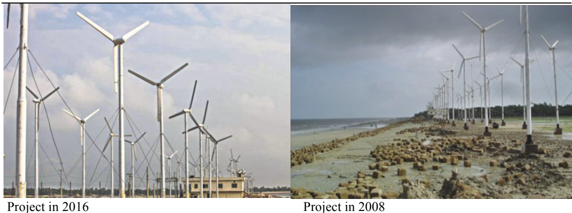
Picture 5.3: Kutubdia wind farm (Source: The Daily Star, 2016)
