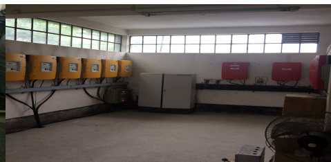
System control room
