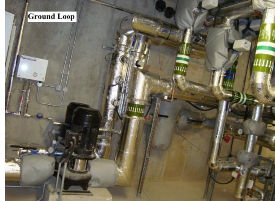
Figure 4 – The Ground Loop Circulating Pump
