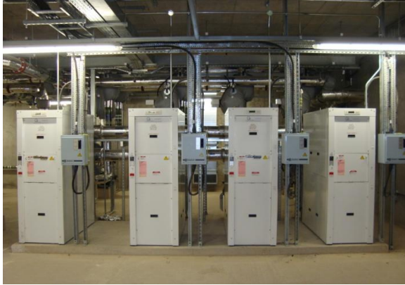
Figure 3 – The Heat Pump Plant Room Installation
