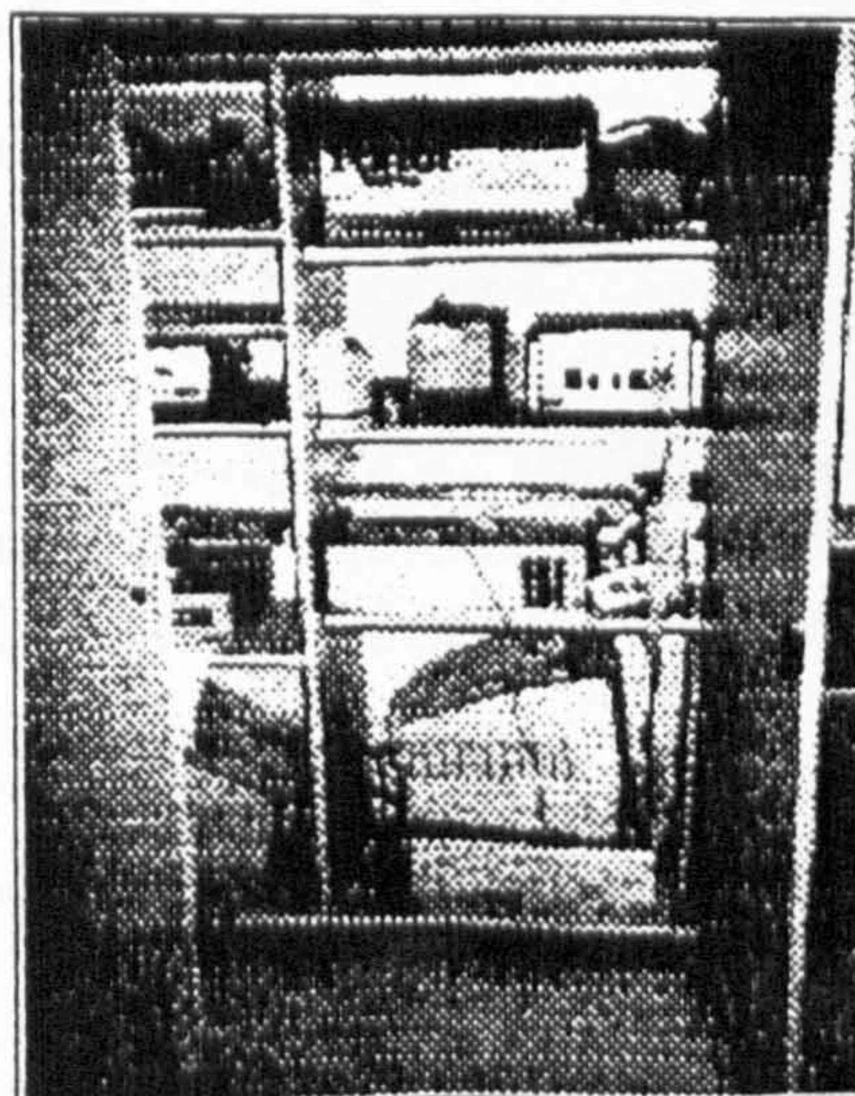
Fig. 4b Bad Example of Standardisation -- Junk behind the door due to lack of transparency
