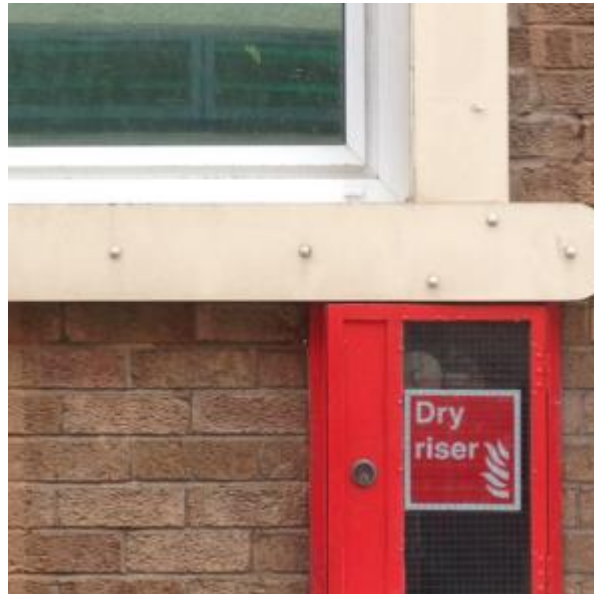
Figure 4.5 : 'Dry riser' on Gateway House. De Montfort University
