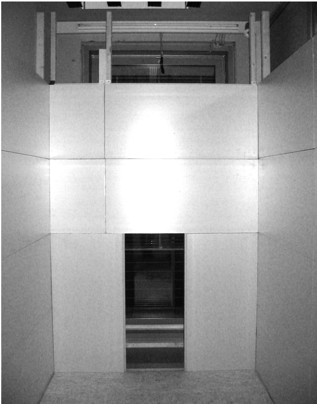
Figure E.3: Outer layer of insulation is installed at rear and side walls. The shown opening was insulated and sealed at the end of construction.
