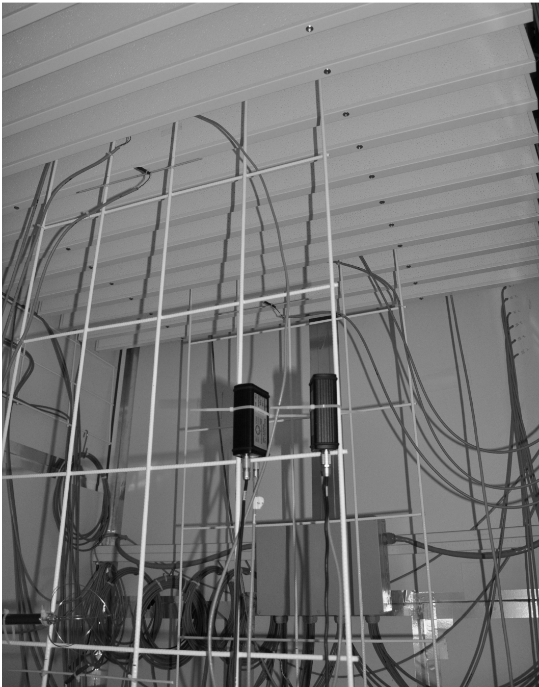
Figure E.12: Rectangular lattice used for installing air temperature sensors and flow sensors in the chamber.
