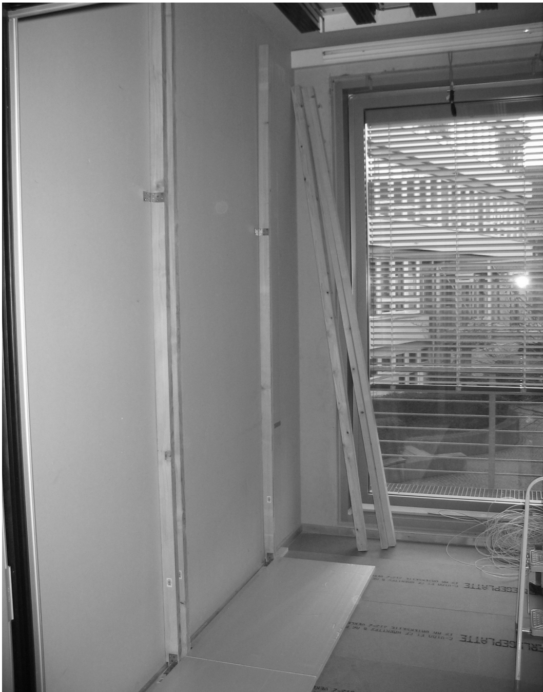
Figure E.2: Inside of the glass compartment. First insulation panels are laid out on the floor, first lumber is installed for construction of the side wall.
