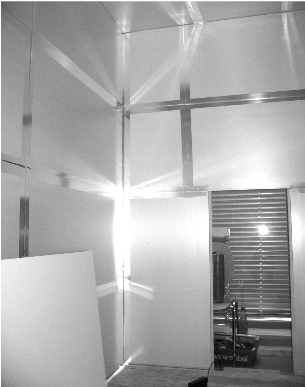
Figure E.4: All joints are sealed with aluminium tape to ensure that leakage is reduced as much as possible.
