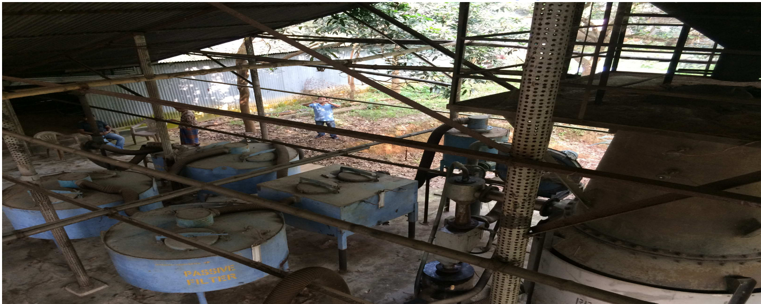
Biomass based RE mini-power plant in Gazipur, Bangladesh
