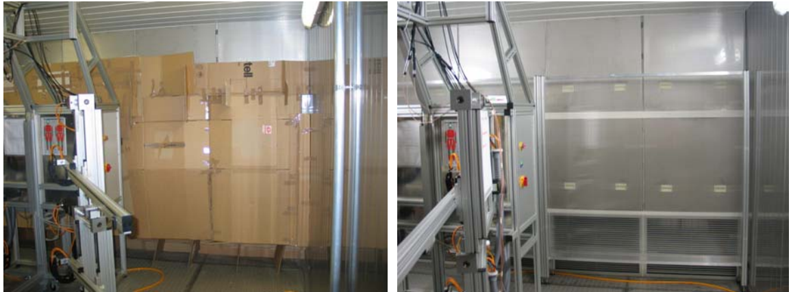
Figure 5.5. The construction of the back partition for homogenous air flow around SAM: full scale model (left) and implemented partition (right).
