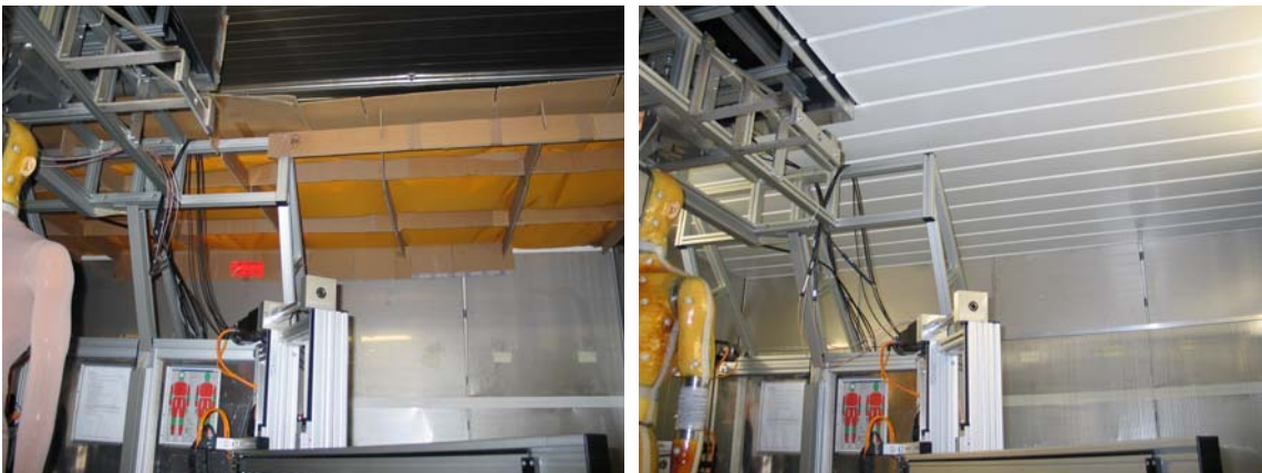
Figure 5.4. The construction of the false ceiling: full scale model (left) and implemented false ceiling (right).
