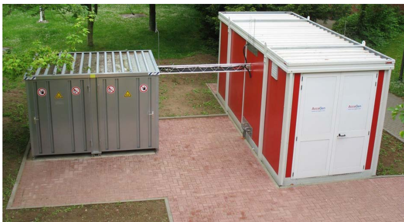
Figure 3-4: The two enclosures of the electrolyser (right) and the gas storage (left).
