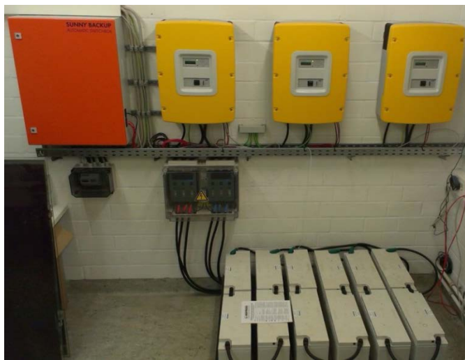
Figure A-3: SMA Backup System composed of the automatic switch box (orange) the three SMA Backup inverter (yellow) and the lead acid battery bank composed of 12 Hoppecke power.com SB 140 batteries (12 V, 142 Ah).
