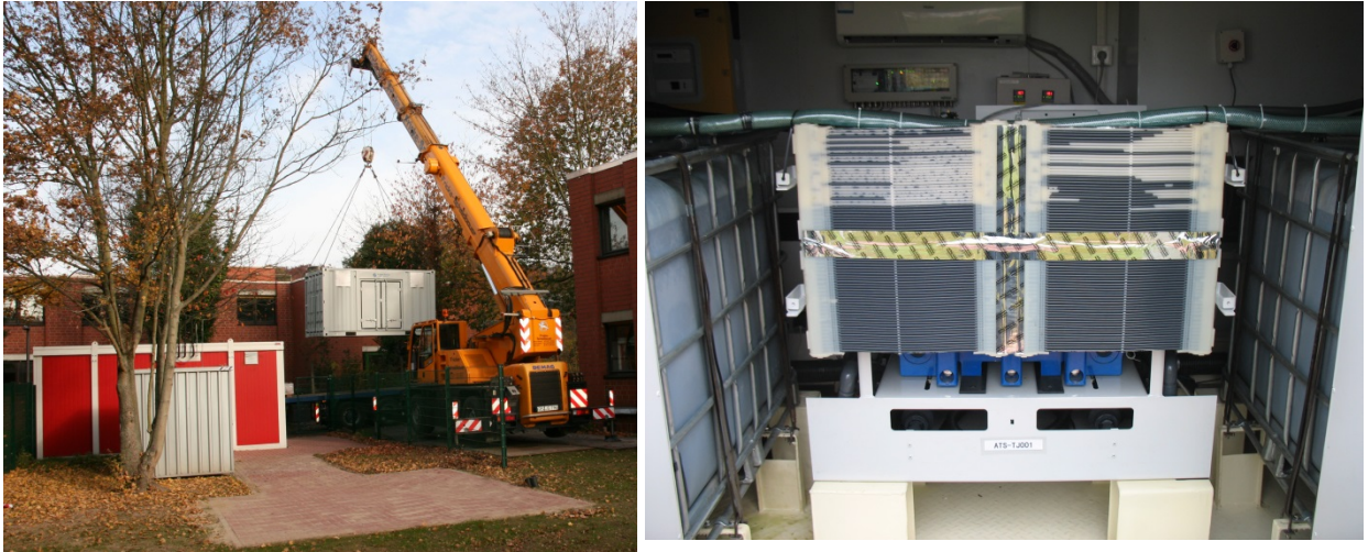
Figure 3-9: Placement of the VRFB container (left). The right hand shows the power module (energy conversion unit, pumps, controller, heat exchanger, etc.) installed inside of the container between the two electrolyte tanks.
