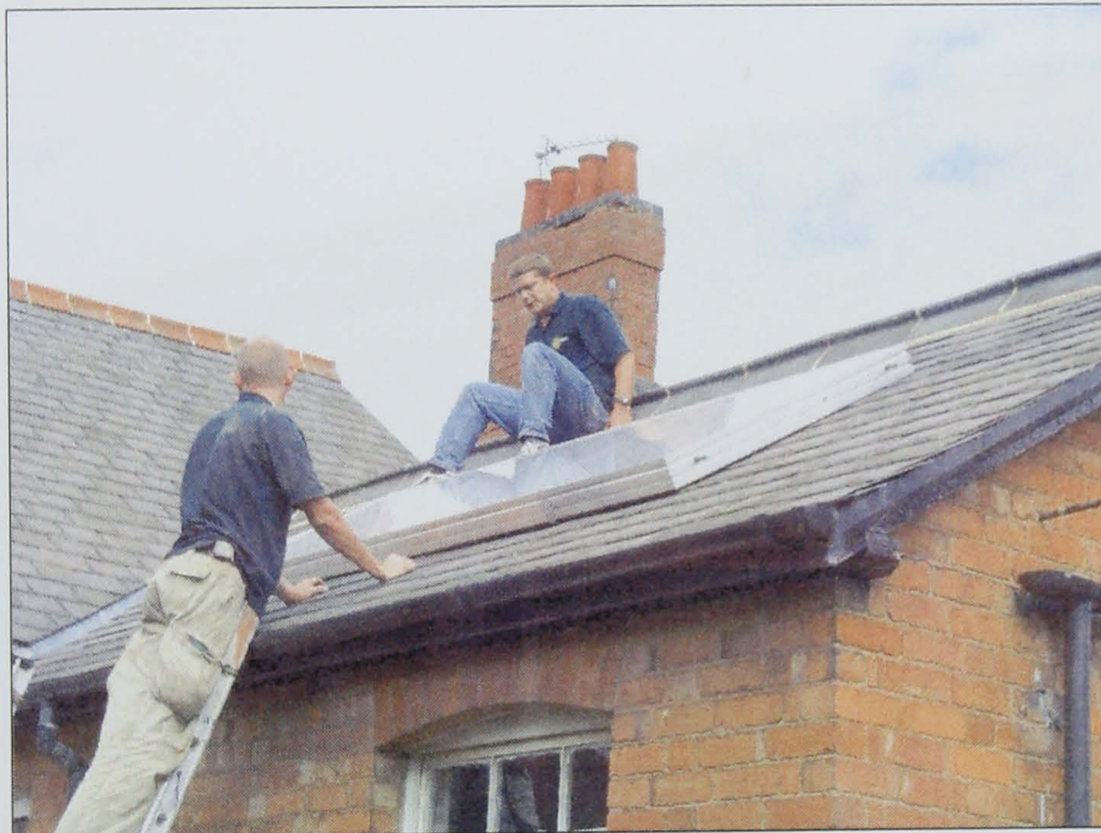
Figure 6. A flat plate solar collector being installed on a house in Melton Mowbray, Leicestershire.
