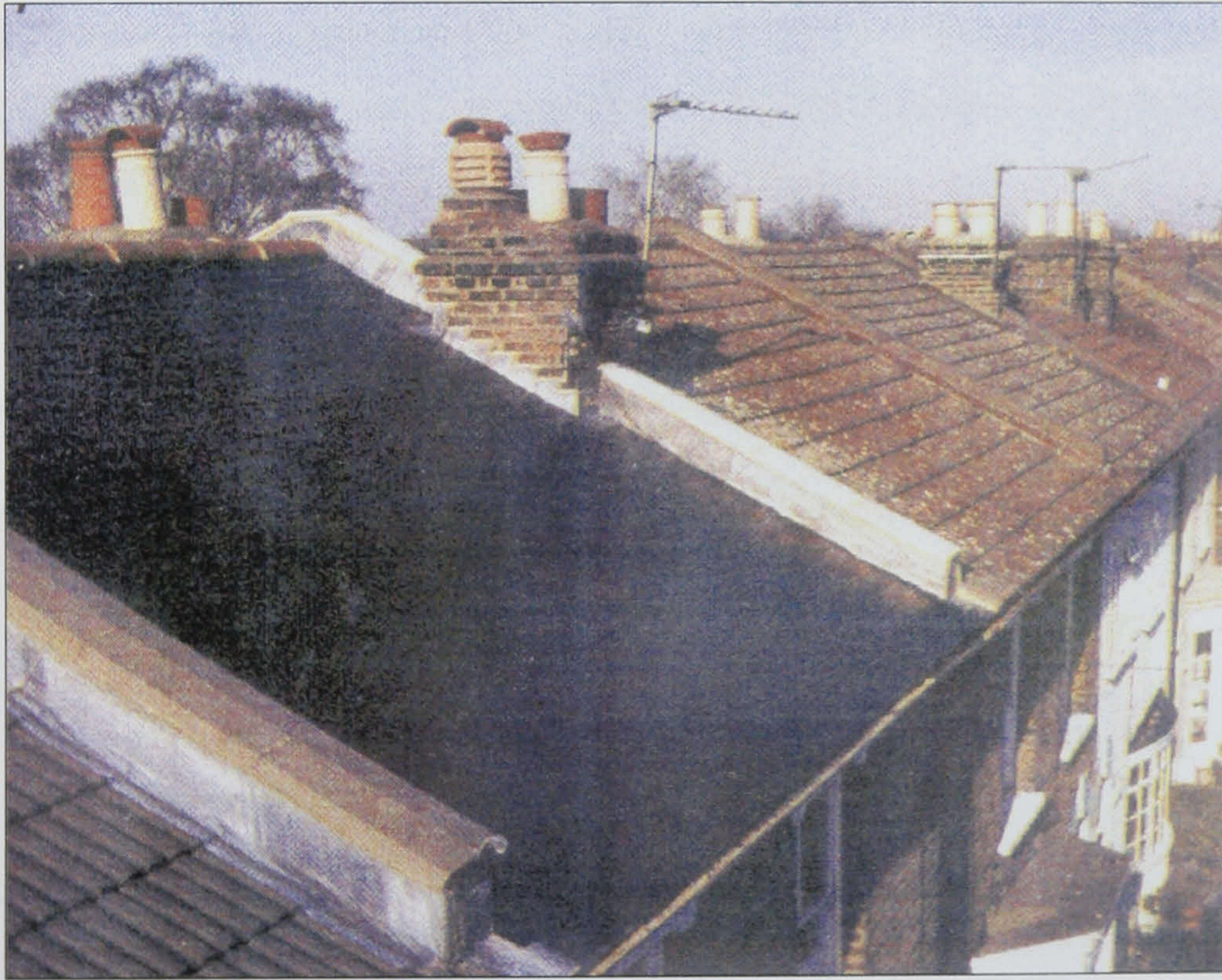
Figure 18. Solar roof tiles installed on a dwelling in the UK. (From Toggweiler, 1999.)
