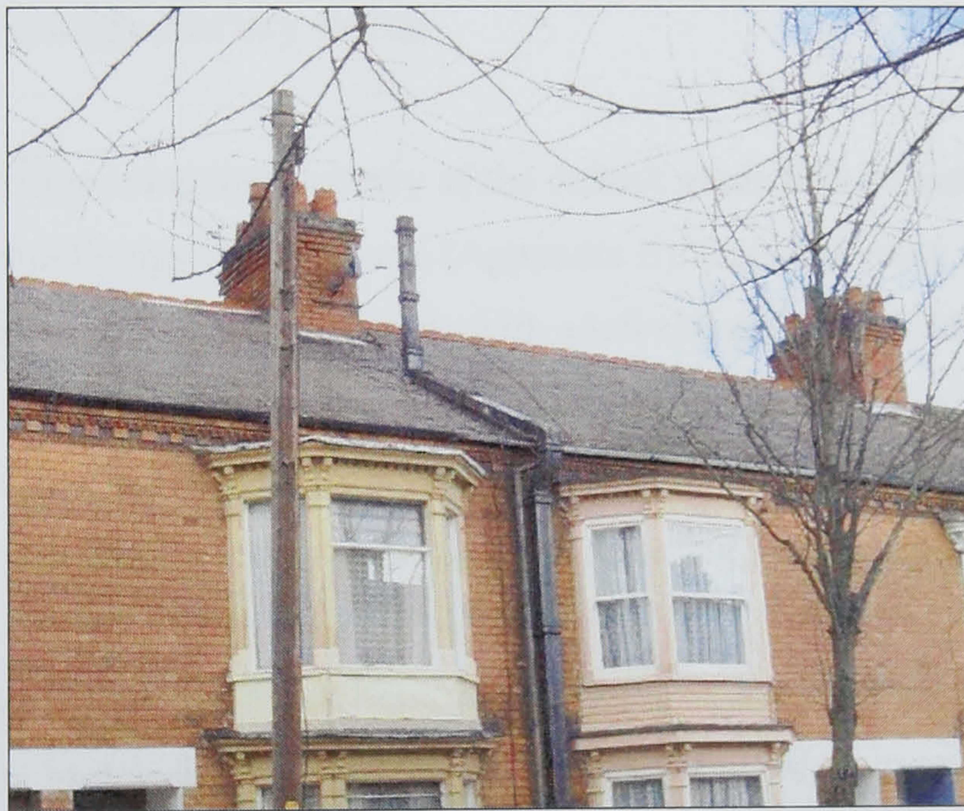
Figure 39. Minor obstructions causing shading problems on a roof.
