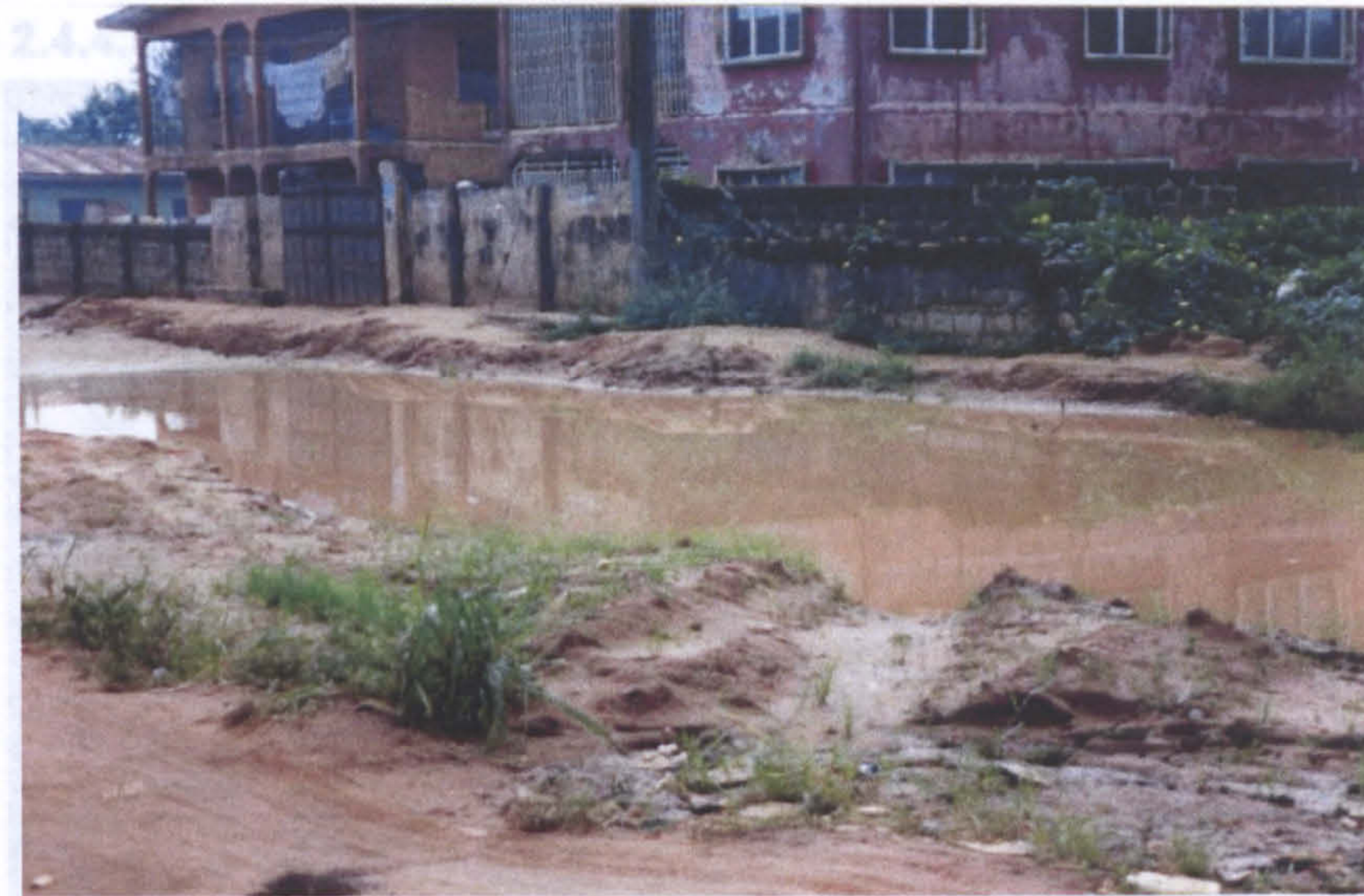
Figure 2.4.4.2.6: Part of a failed portion of a road in Ojota, Nigeria (2004)
