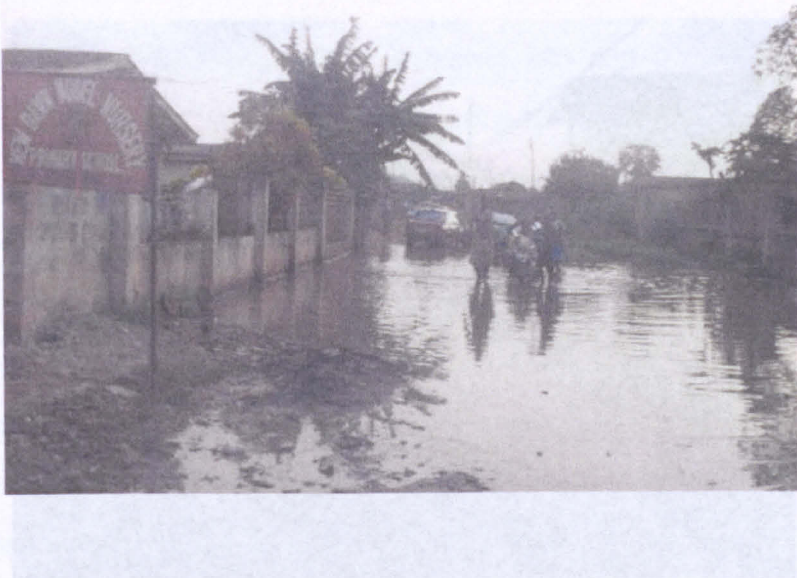
Figure 2.4.4.2.5: A failed portion of Uwanota road in Benin City (2005)
