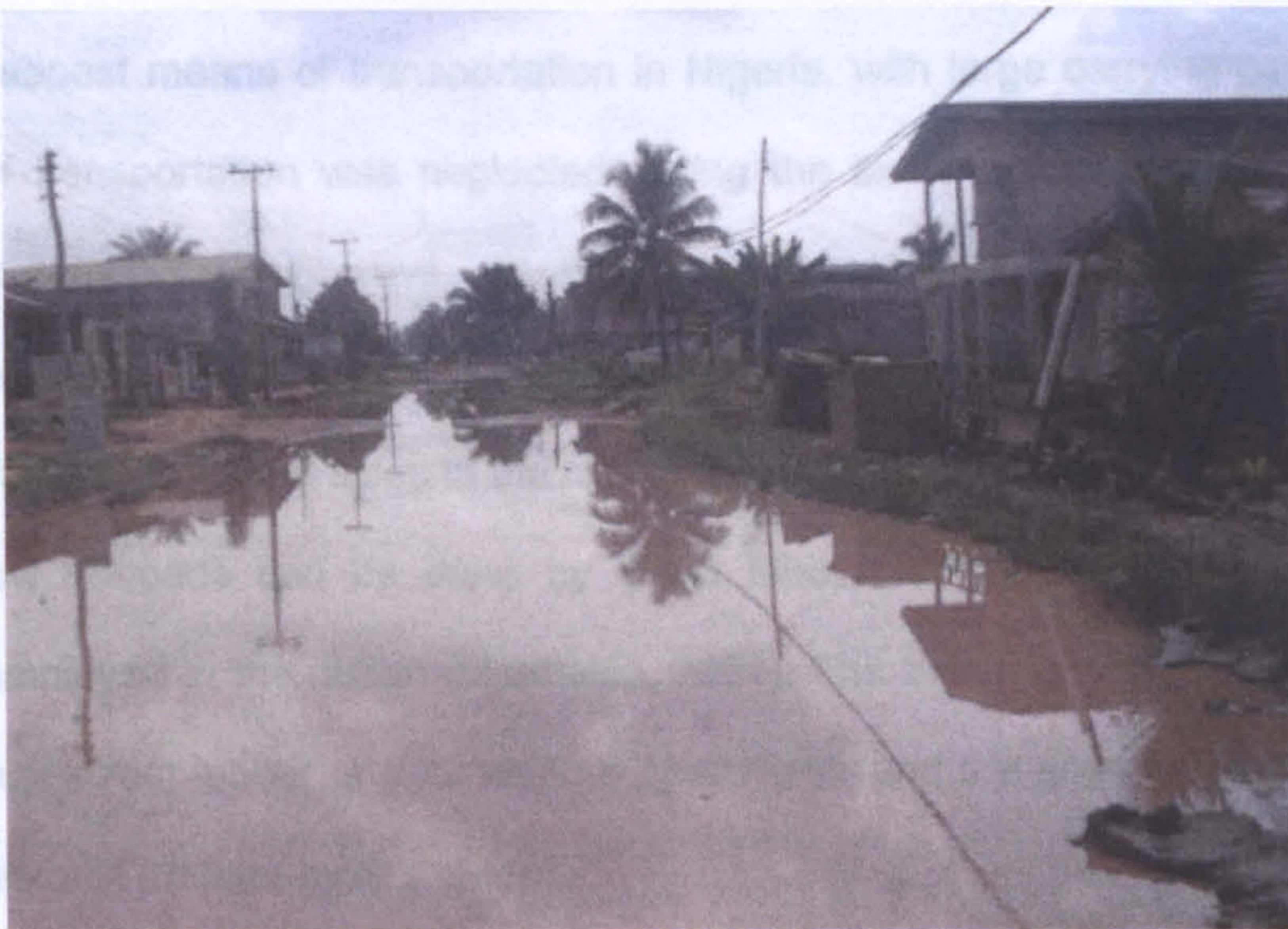
Figure 2.4.4.2.5: A failed portion of Uwasota road in Benin City (2005)
