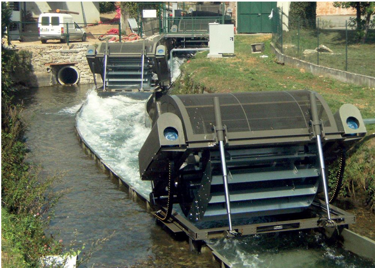
Figure 1. New 32 kW waterwheels at Canavese Canal, Turin
