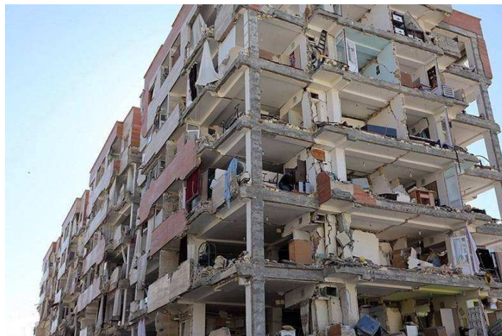
Figure 1. Extensive damages to exterior and facade walls of buildings despite the acceptable performance of the lateral load-bearing systems in the Kermanshah earthquake, 2017
