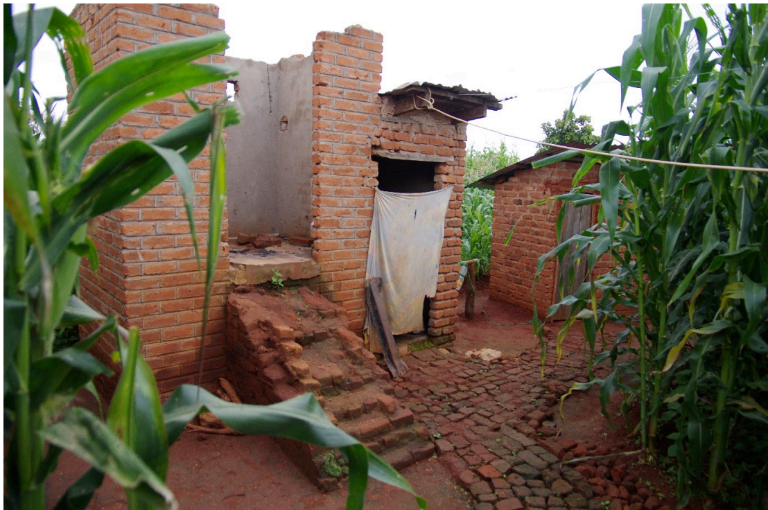
Photograph 1. Abandoned Skyloo and latrine used instead (right)
