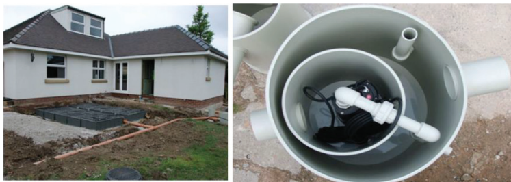
Figure 1. Left: Skeletanks® in place and connected together. Right: lightweight pump chamber.
