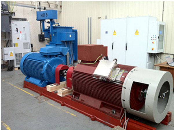
Fig. 2 250 kW D400 BDFM (right front) on test bed
