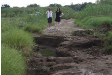
Figure 16: Cheryl McEwan and Alex Hughes survey the damage wreaked by the 2011 floods. Here the waters have washed away part of a dirt road.
