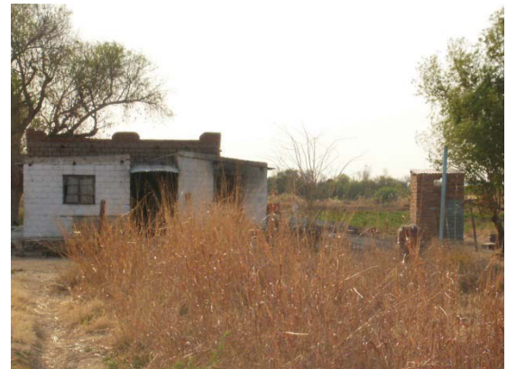
Figure 20: A dwelling on South Island which still has a hole in the roof caused by hail in 2002. Water has to be collected from an open channel nearby.
