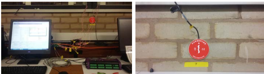
Figure 8: Non-invasive monitoring equipment installed.
