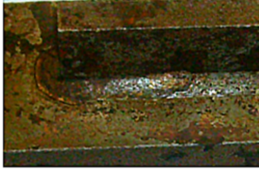
Fig. 3: Close-up of area of interest of ultrasonically peened fillet welded specimen after removal of rust
