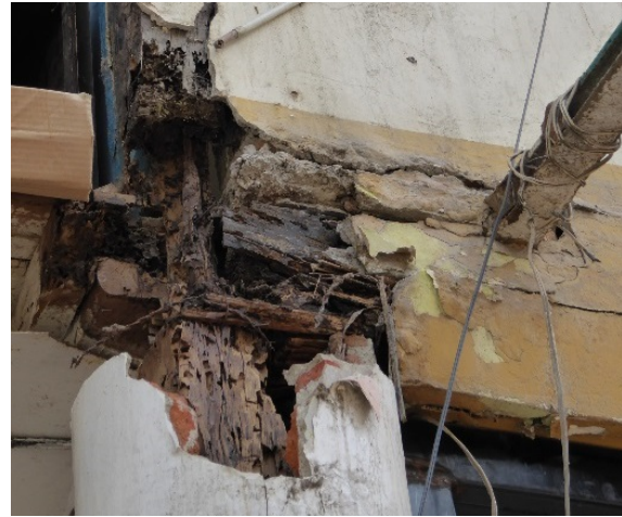
Figure 47: Rot damage to timber in traditional bahareque housing, Ecuador (Kaminski, 2016)
