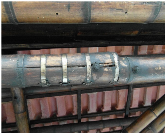
Figure 73: Steel pipe ties used to strengthen bamboo after it had split, Colombia (Kaminski, 2016)
