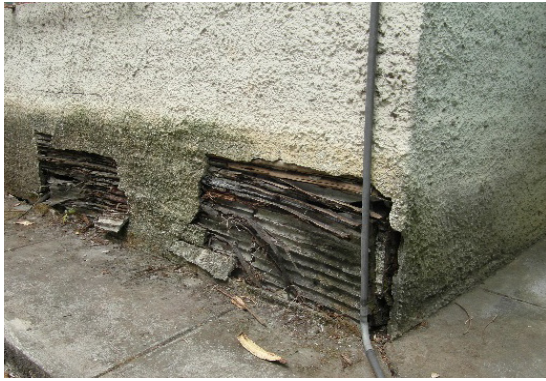
Figure 40: 100% section loss of cane to the base of walls, Costa Rica. Note the mould visible at the base of the walls due to splashback from the roof. The cement and paint is clearly not sufficient protection under driving rain (Kaminski, 2016)
