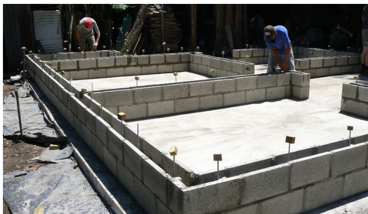
Figure 60: Example of simple upstand of engineered bahareque housing in El Salvador, consisting of two courses of reinforced blockwork, totalling 400mm high from the foundation
