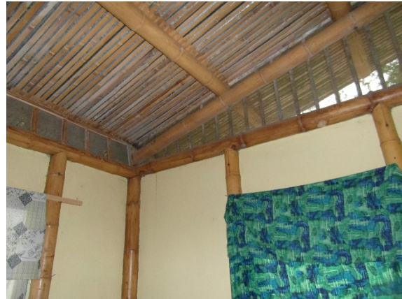
Figure 17: Interior view of PNB house in Milano, Costa Rica – photo taken at 20+ years since construction (Kaminski, 2016)
