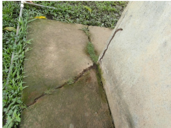
Figure 37: Subterranean termite shelter tube emerging from crack (Kaminski, 2016)
