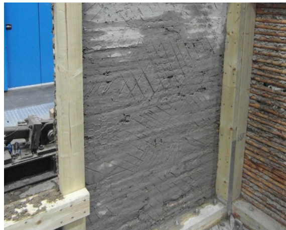
Figure 74: Maintaining a good bond between subsequent cement mortar render layers by roughening the previous layer while still setting (Kaminski, 2016)
