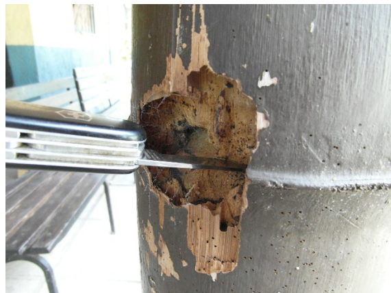
Figure 35: Severe termite damage in bamboo, Costa Rica. The small round black drywood termite droppings are just visible (Kaminski, 2016)
