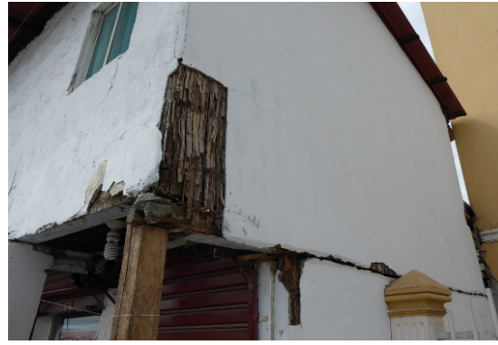
Figure 41: Spalling of render after earthquake, revealing rotten bamboo esterilla below, Ecuador (Kaminski, 2016)
