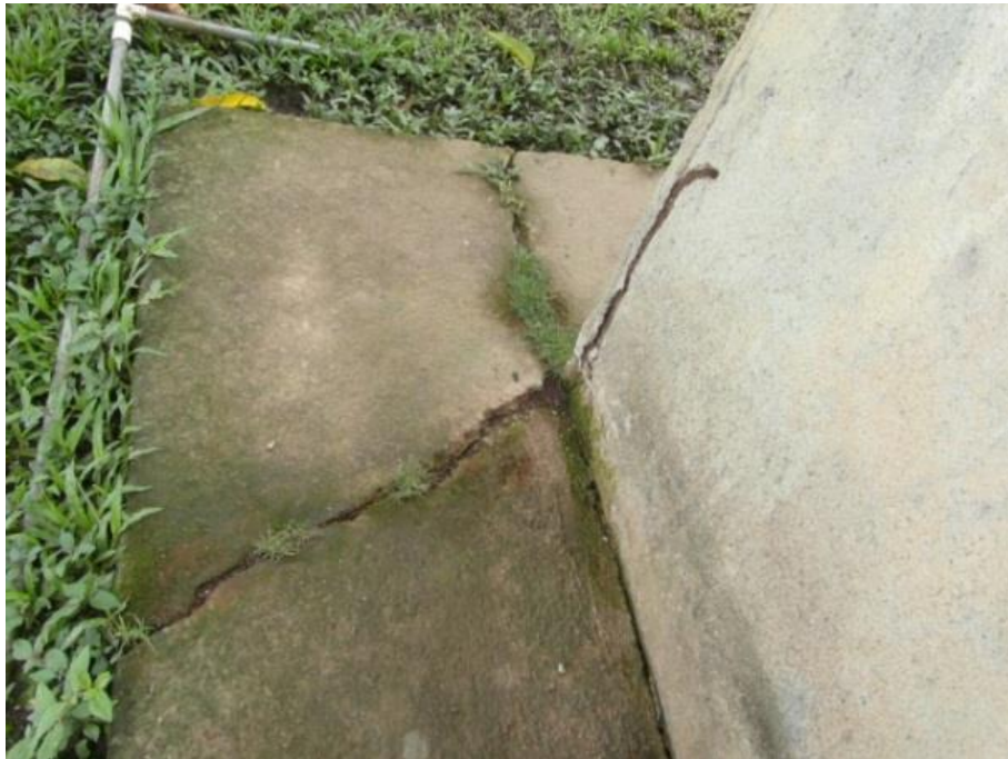
Figure 4: Subterranean termite shelter tube emerging from crack 3
