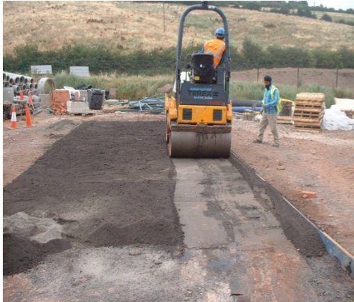
Fig 4. CEM0 trial with a mix without aggregate. This semi-dry paste was laid in a 100mm layer on top of soil that had been previously stabilised using CEM0.
