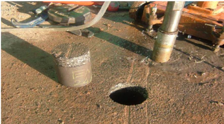
Figure 124. Core sample taken from the lower part of trial road at the King's Mill Hospital site.
