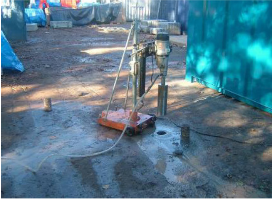
Figure 128. Core sample taken from middle and end part of the trial car park at the Lowdham Grange site .
