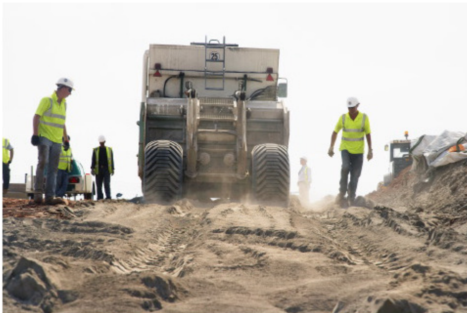
Figure 106. Blending the mixture of soil and binder using the rotavator (rotavator moving into position).
