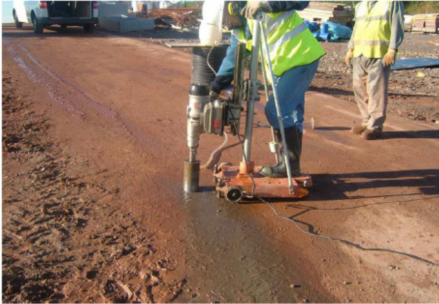
Figure 123. Coring machine used to drill the cores at the King's Mill Hospital site.
