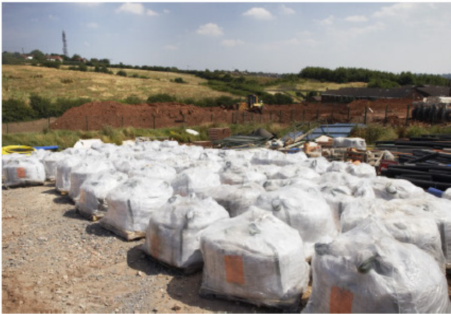
Figure 86. 1000-kg bags of blended powder ready to use (King's Mill Hospital site).
