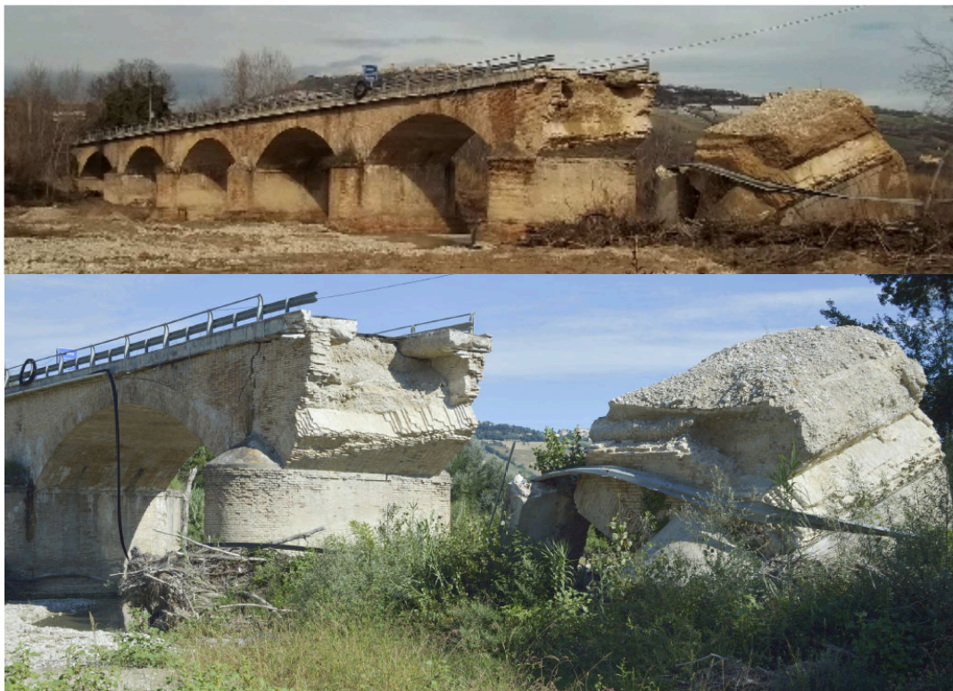
Figure 1. Global view of the bridge after the pier collapse during the 2013 flood and detail of the scour-induced down-stream rotation of the pier.
