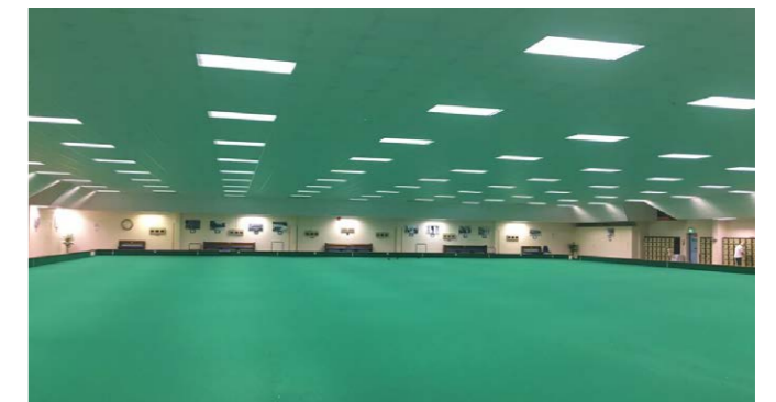
Figure 5 - LED lights installed in a bowling club (BHESCO, 2019a)
