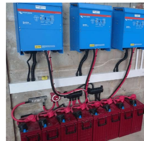
Figure 3 – Battery storage at a Golf Club (Curtis, 2018a, 2018b)
