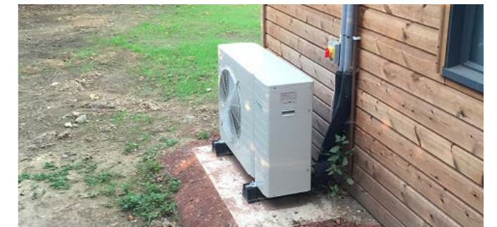
Figure 4 - An air-source heat pump at The Montessori School (BHESCO, 2019a)
