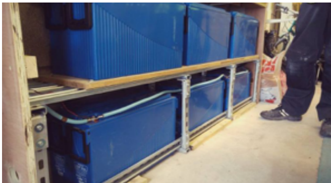
Figure 5 -First Gwent Energy Battery Installation 2015 (Gwent Energy CIC, 2019f)
