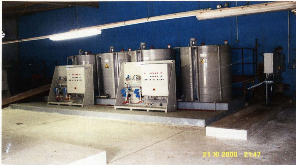
Figure 1.4 – Photographs of chemical dosing units of the Tajoura SWRO desalination plant.
