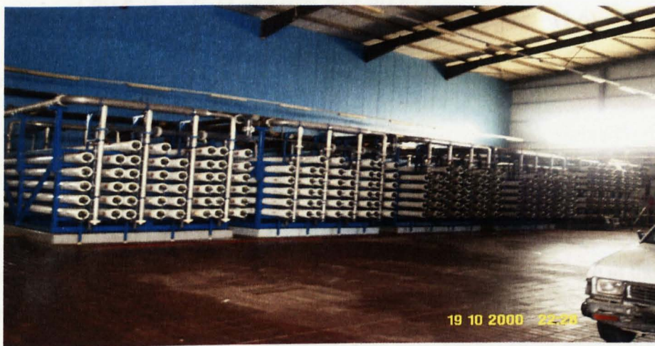
Figure 1.7: Photograph of reverse osmosis membrane trains of the Tajoura SWRO desalination plant.
