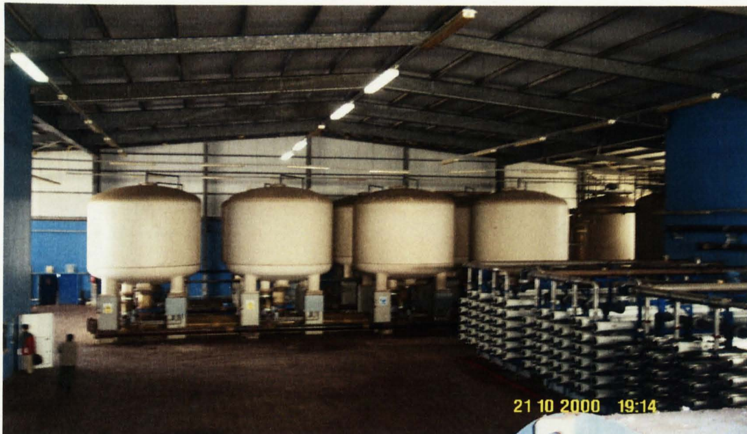
Figure 1.5 – Photographs of multimedia filters of the Tajoura SWRO desalination plant
