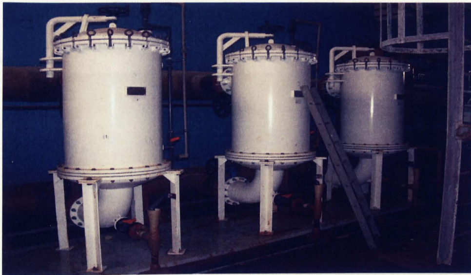
Figure 1.6: Photograph of cartridge filters casing of the Tajoura SWRO desalination plant.
