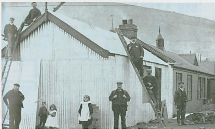
Photograph 8.9. The Derwent Canteen during construction work to extend it. Brian Robinson Collection
