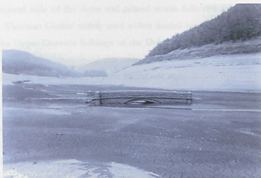
Photograph 8.20. A 19 th century road bridge across the River Derwent lies submerged in the silts of Derwent Reservoir
