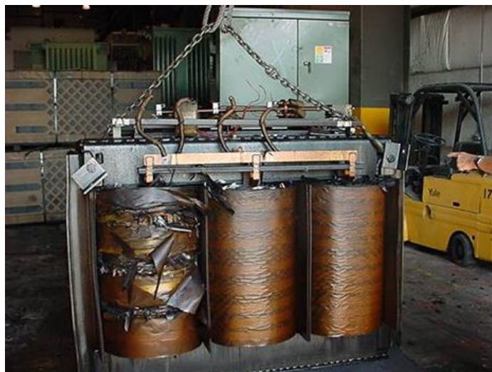
Figure 2.2. Power transformer failure ( http://electrical-engineering-portal.com ).
