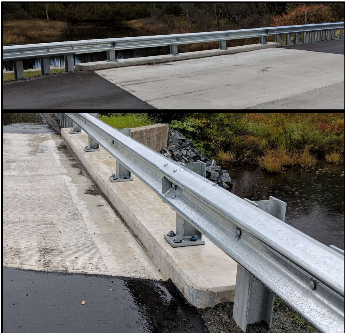
Figure 3: Example of a concrete bridge curb. This curb is approximately 29 feet long and is located on NH 113 in Grantham, NH.
