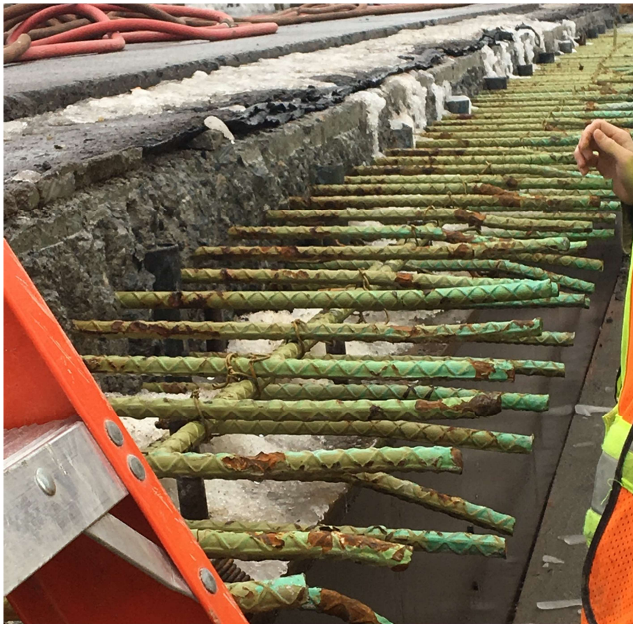
Figure 4: Exposed rebar extending out from a bridge deck after the former curb had been demolished.
