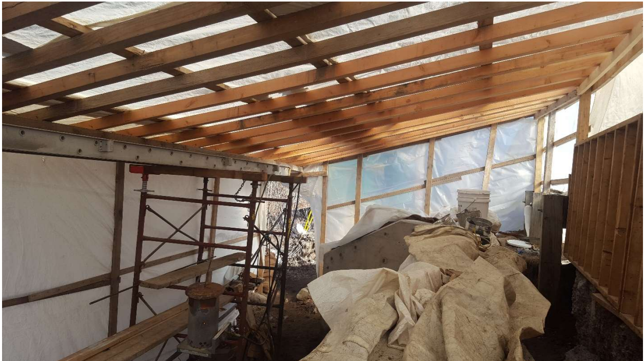
Figure 8: A heated enclosure constructed over a bridge to prevent concrete from freezing during curing.
