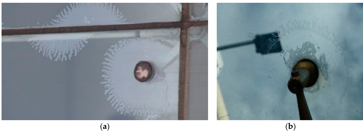
Figure 6. Examples of severe delamination in LG member, in the region of point mechanical restraints. Reproduced with permission from (a) [36] and (b) [37].
