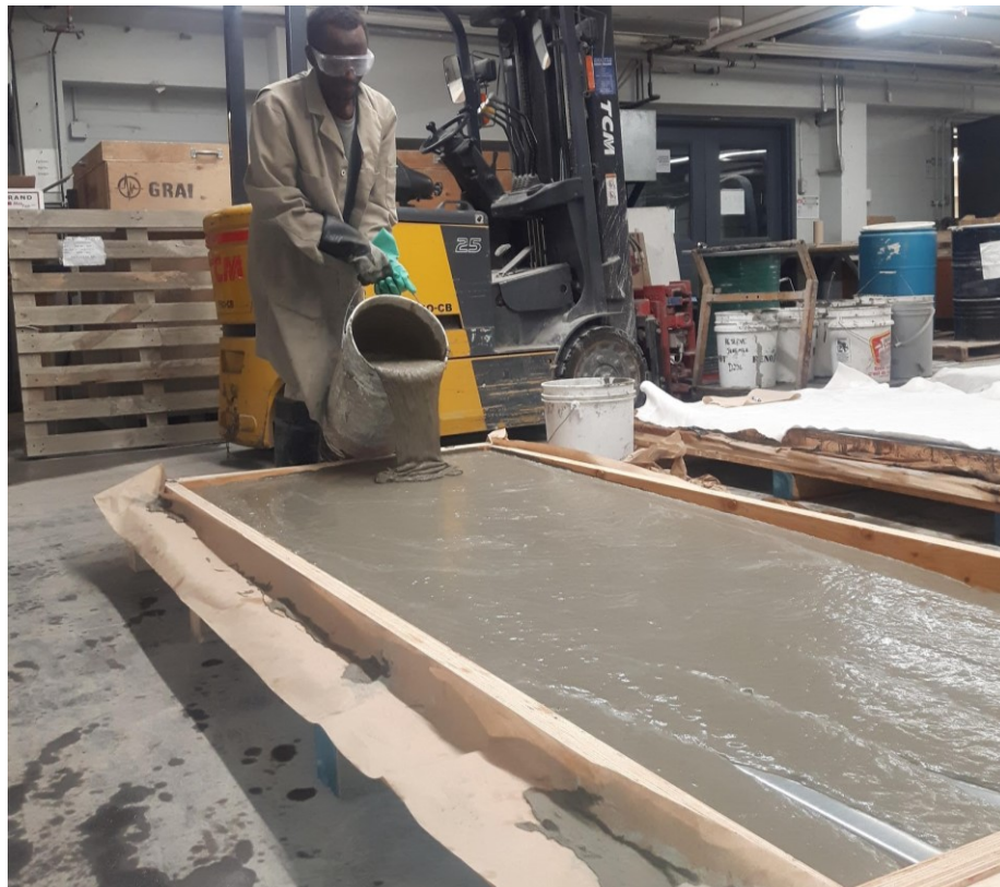
Fig. 4. Casting of SHCC slabs: The figure depicts the exceptional texture, rheology, and self-consolidating ability of nHVGP-SHCC. The figure shows an SHCC slab where no WWM are used.
