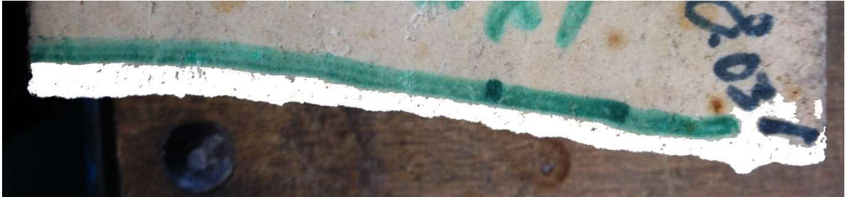
Figure C1 – Crack profile highlighted.
