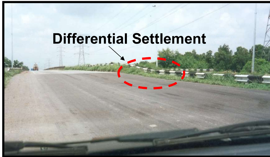
Figure 1.3: Undulating road at structure approach
