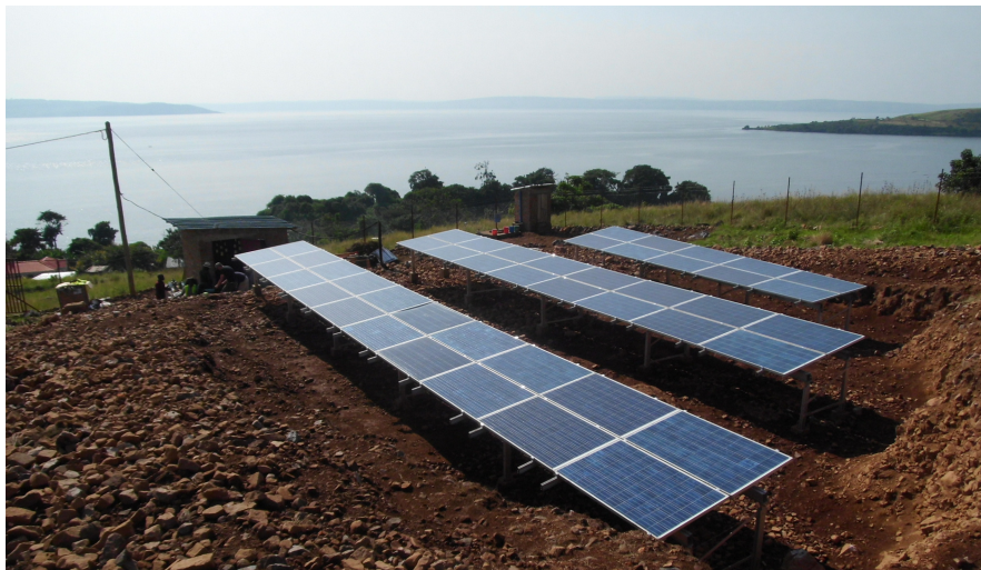
Figure 5. System overview picture with photovoltaic installation in the foreground and the battery powerhouse on the left. For the solar modules, the area was leveled out to achieve good alignment. The visible power pole represents the connection point to the external stand-alone grid. For security reasons, the property is fenced in. This kind of project in the vicinity of water bodies also requires sanitary facilities, which can be recognized in the center of the picture. In the distant background with a view to the west, the mainland is already noticeable.
