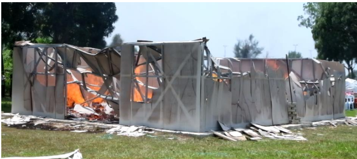
(c) Deformed shape of structure at 38 min
