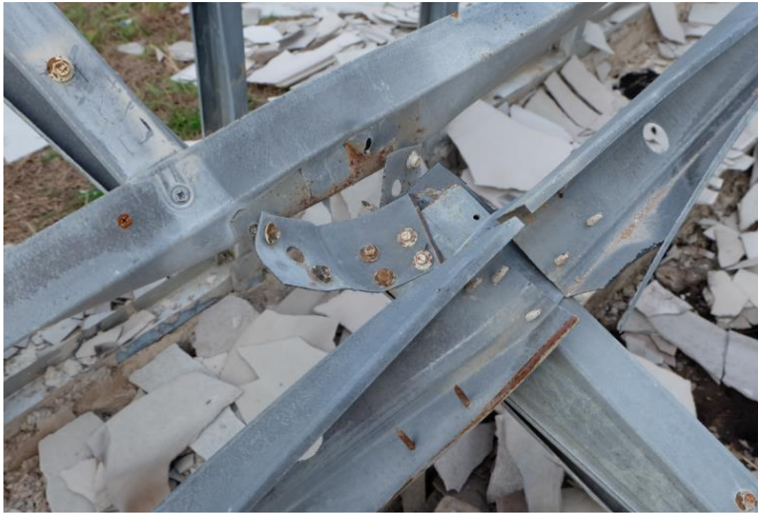
Fig. 12: Eave connection failed
