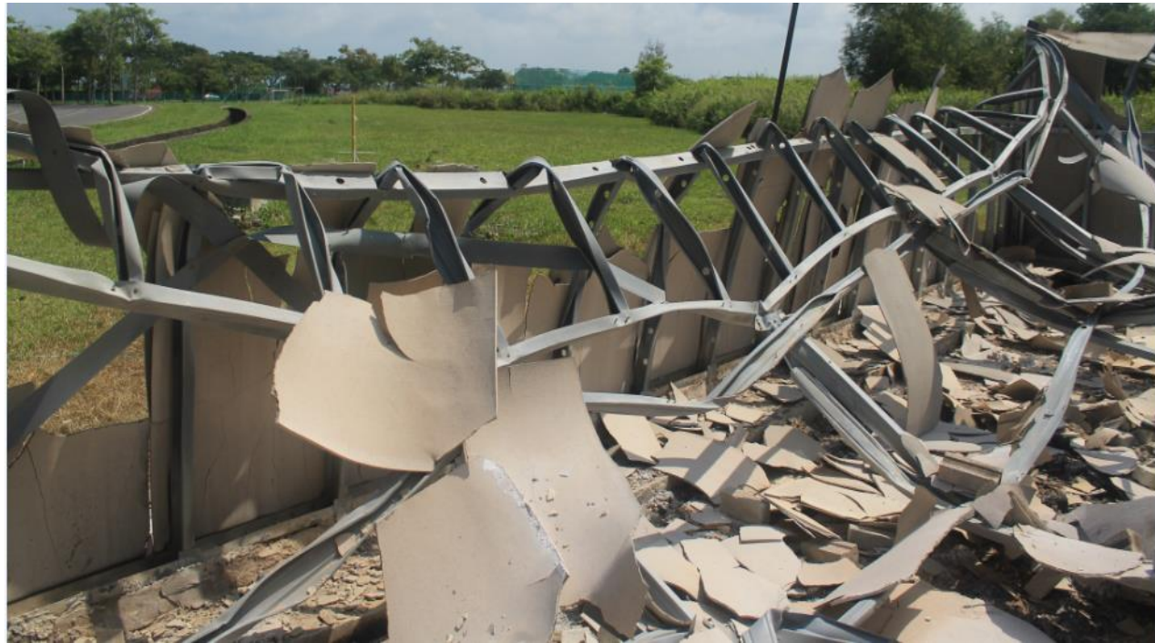
(a) Final deformed shape of north wall
