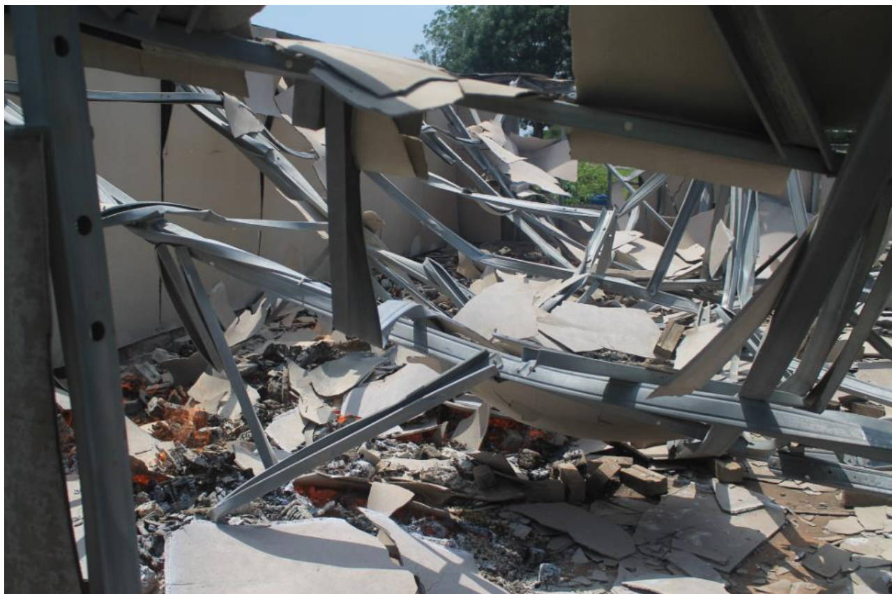
(c) Final deformed shape of the roof truss
