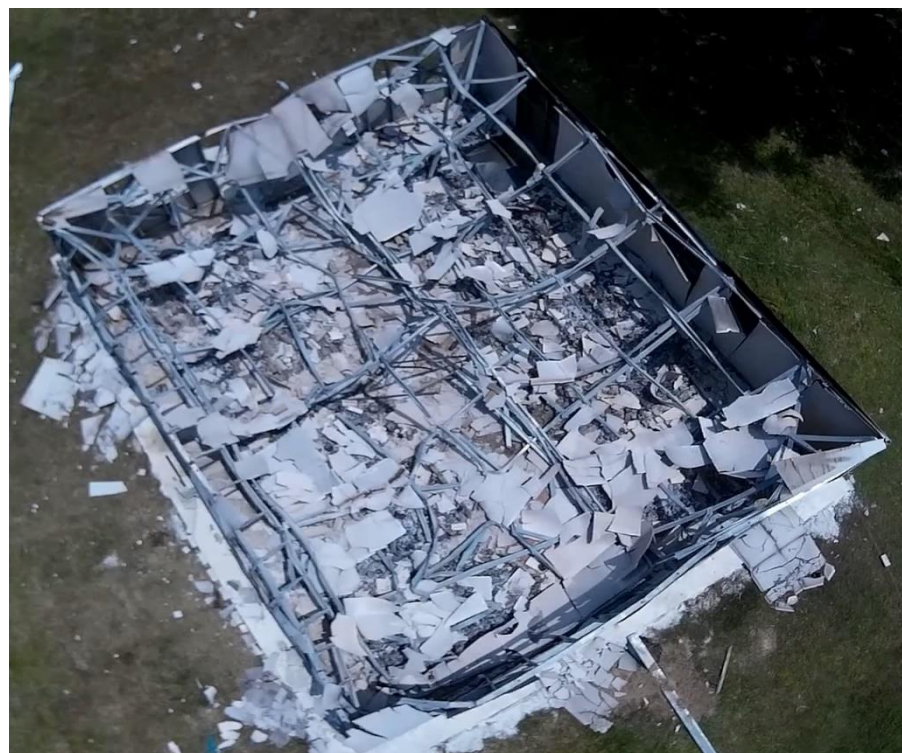
(d) Final deformed shape of the cold-formed steel building at the end of fire test Fig. 9: Failure of the CFS building at different time during the fire test
