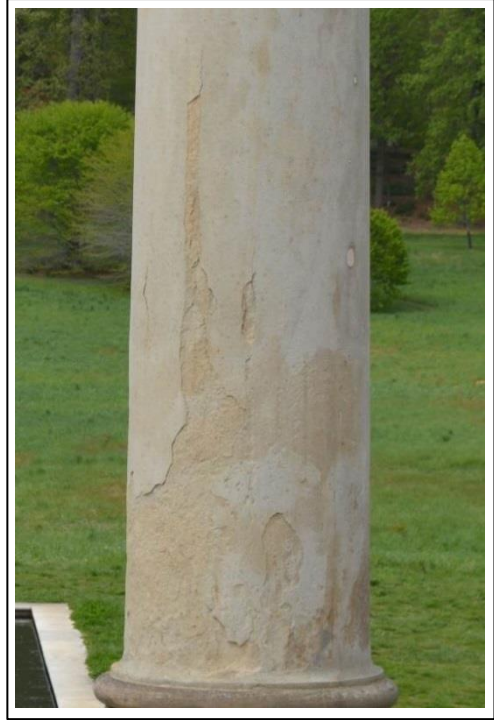
Fig. 4: The lower shaft of column L20 has the highest contour loss, extending more than six feet; a detached area reaches even higher. The area of detachment can be seen on the left.
