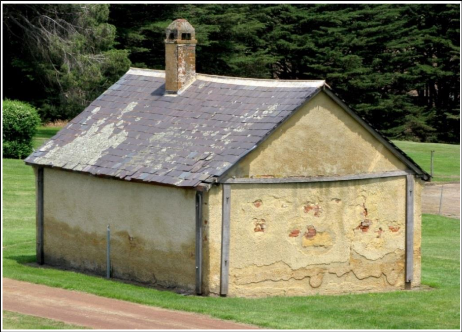
Fig. 2: Woolmers Estate blacksmith's shop from the north. Failed rendering (harling) on the northwest wall (to the right) is allowing penetrating dampness to carry salts through the 350 mm brickwork to the interior (see Figure 3).
