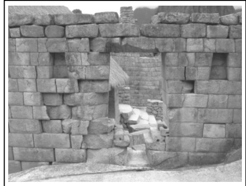
Fig. 4: Severe damage of the northern opening area.
