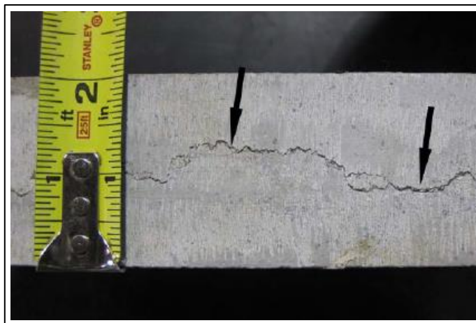
Fig. 3: Microcracks parallel to stone face.
