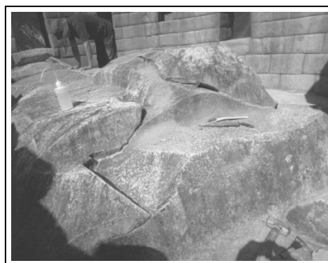
Fig. 7: Decay of natural rock pedestal.
