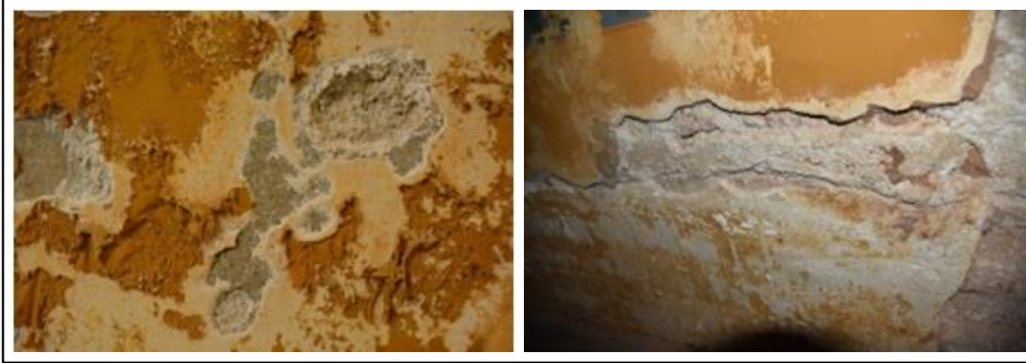
Fig. 2: Exfoliation of inner stucco (left) and middle-layer mortar with salt crystallisation (right)
