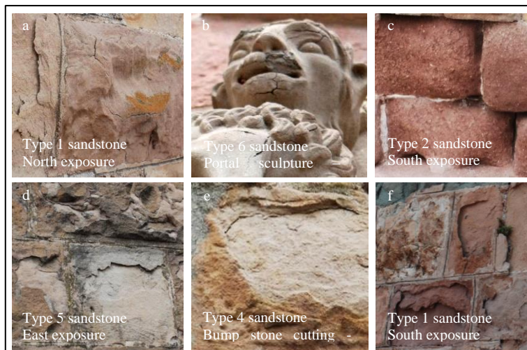
Fig. 2: Details of craquele, scaling and granular disintegration patterns.
