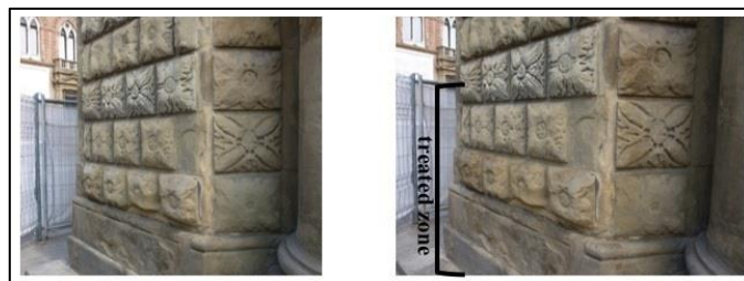
Fig. 7: The sandstone before (left) and 30' after the \text{TiO}_2 application (right).
