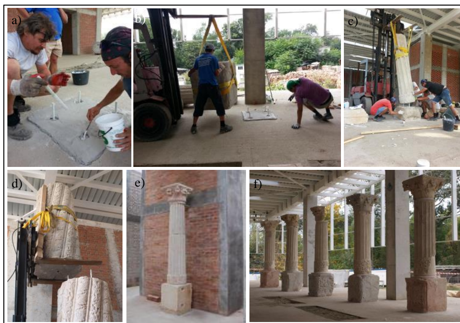
Fig. 5: Installation of the columns: a and b) Bottom pin structure, c to e) Assembly of the decorated stone block to columns in the Royal House; f) Columns of the veranda.
