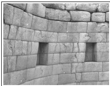
Fig. 5: Cracks and detachments.
