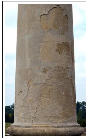
Fig. 6: Same location as the previous in 2013, showing an estimated 10-15% additional contour losses after 25 years.
